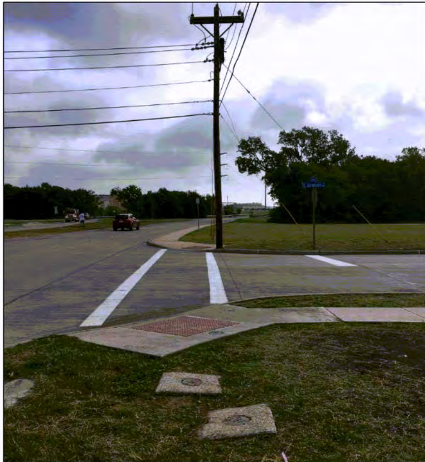
Figure 31: Non-Compliant Pedestrian Ramps crossing east leg of New Hensley Ln at Woodbridge Pkwy
