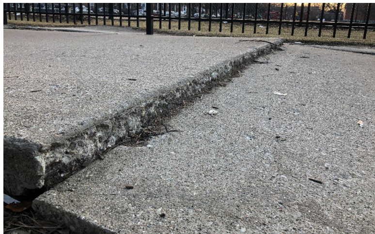
Example of a Sidewalk Requiring Repair
