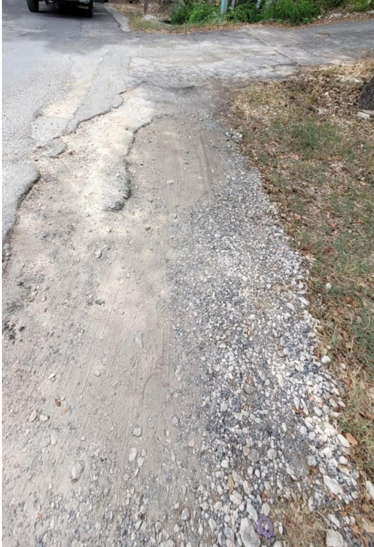
4 Tremont Trace – Before (Asphalt Driveway & Approach)
