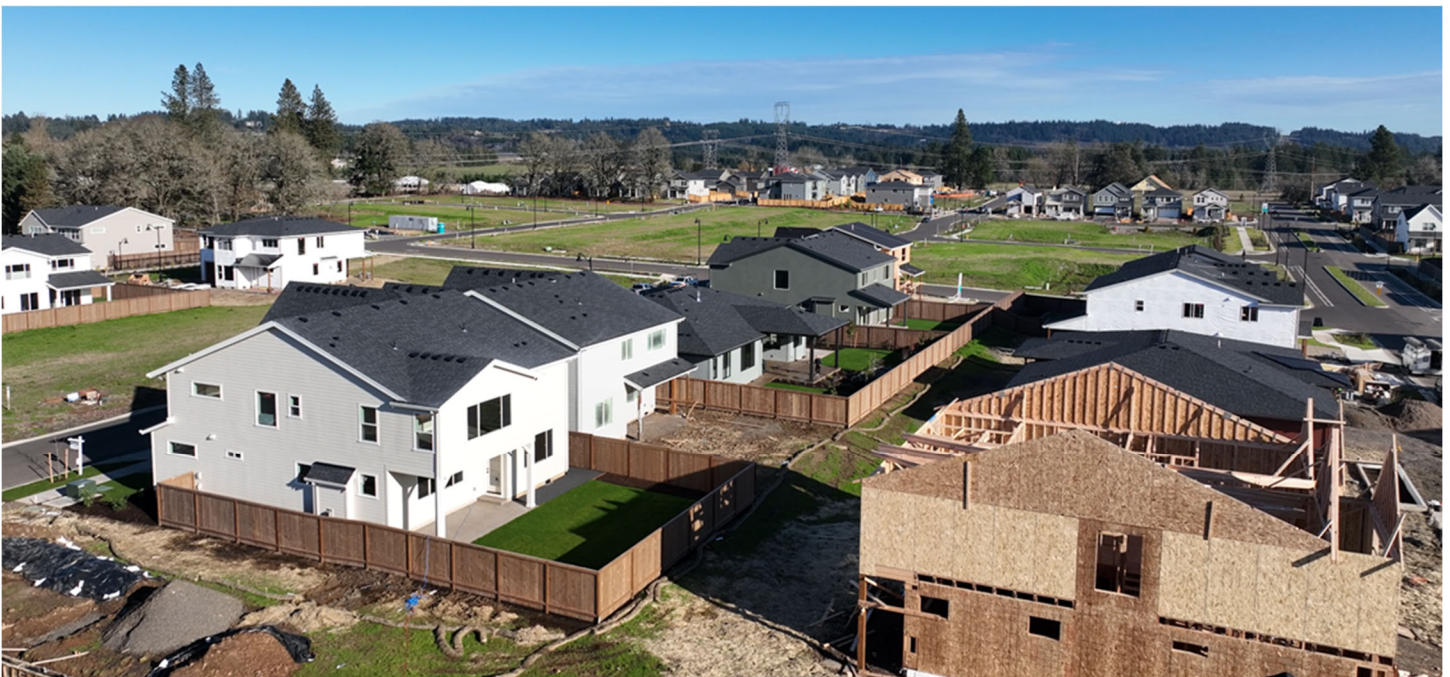
Construction continues at Frog Pond Crossing, Frog Pond Oaks and Frog Pond Vista
