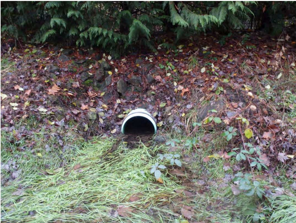
Photo 6 Partly submerged 18-inch CCP contributing culvert
