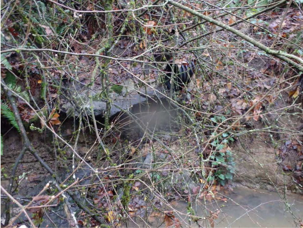
Photo 16 Perched Culvert on Right Bank
