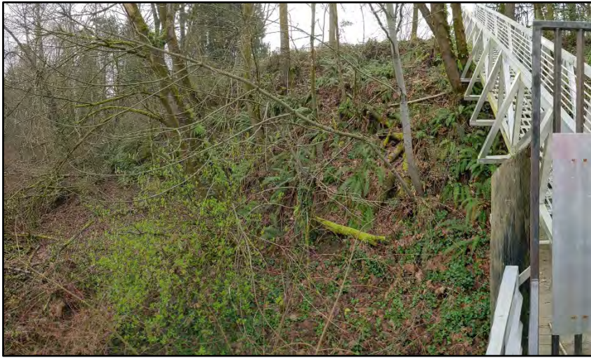
Photograph B-5. Photograph looking southeast upslope. Trees against gangway to be removed visible. Photograph taken 3/7/2022.
