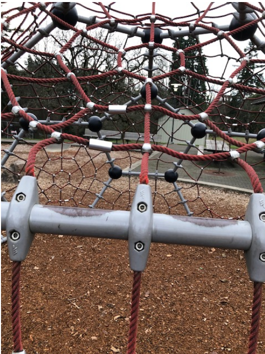
Exposed metal on posts (high usage/age)
