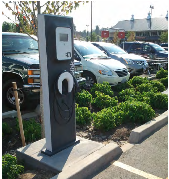
The recent Fred Meyer near the I-5/Wilsonville Road Interchange provides two electric vehicle charging stations for patrons to use for free to charge their vehicles while shopping.
