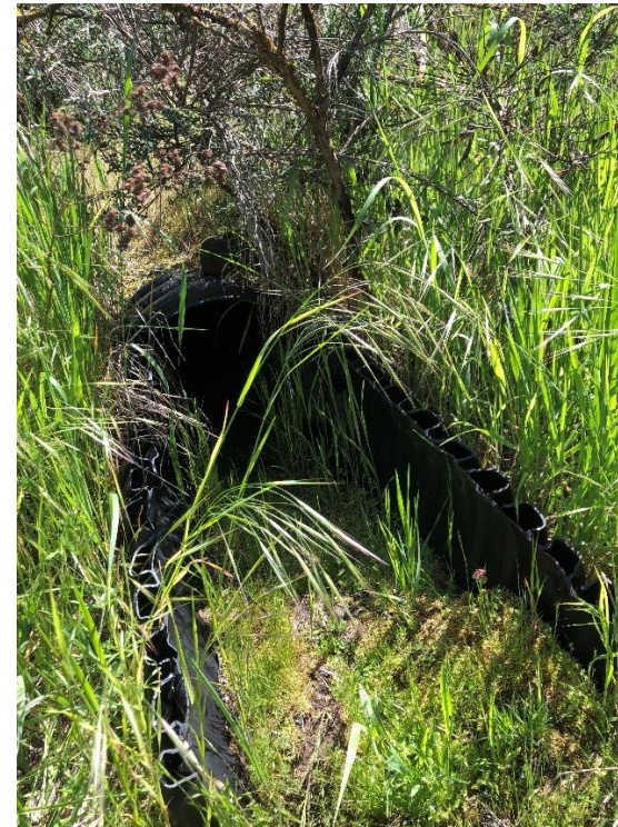
Garden Acres Pond Existing Inflow Pipe (May 2023)
