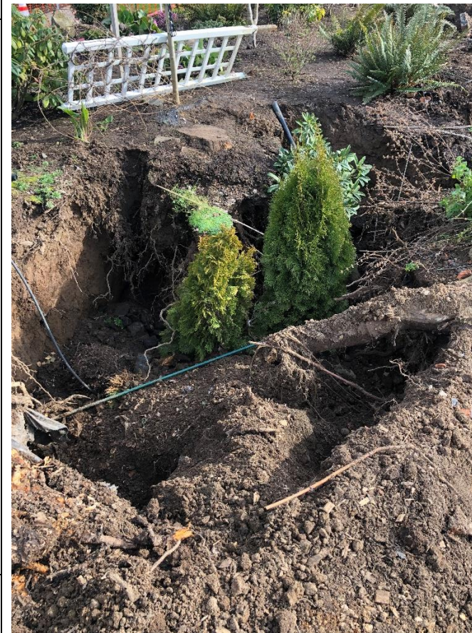
Sinkhole observed at upstream end of Miley Road alignment
