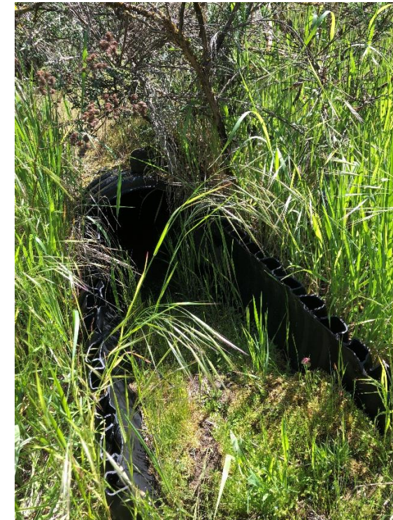
Garden Acres Pond Existing Inflow Pipe (May 2023)
