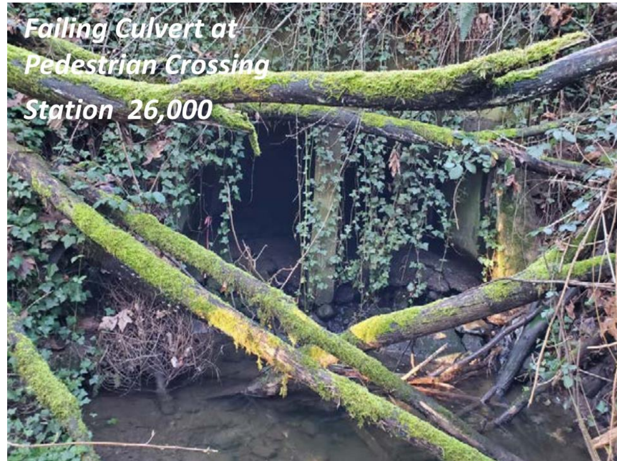
Failing twin 5 ft x 5 ft culverts under pedestrian crossing looking upstream (Source: Geomorphic Stream Assessment, Waterways Consulting, May 2022)
