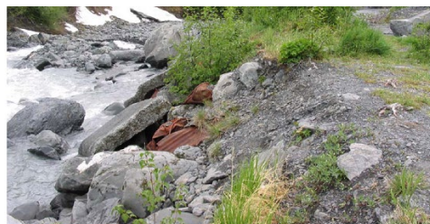
Figure 4. Downstream end of Whittier Creek Dike looking downstream. Note lack of vegetation on bank and debris used as bank protection.
