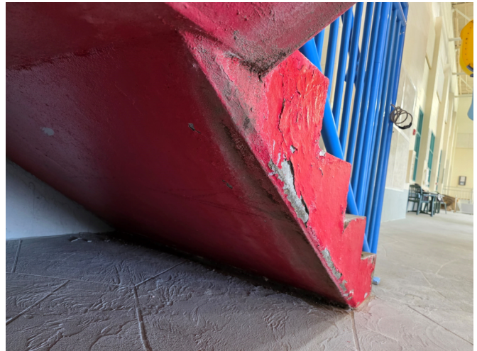
6. FLAKING/WORE PAINT AND FINISH
