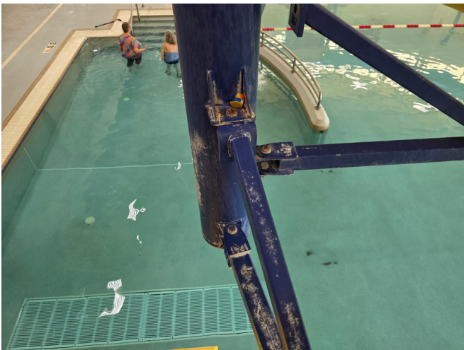
5. FLAKING/WORE PAINT AND FINISH
