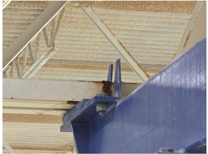
16. CORROSION ON ROOF/CEILING SYSTEM
