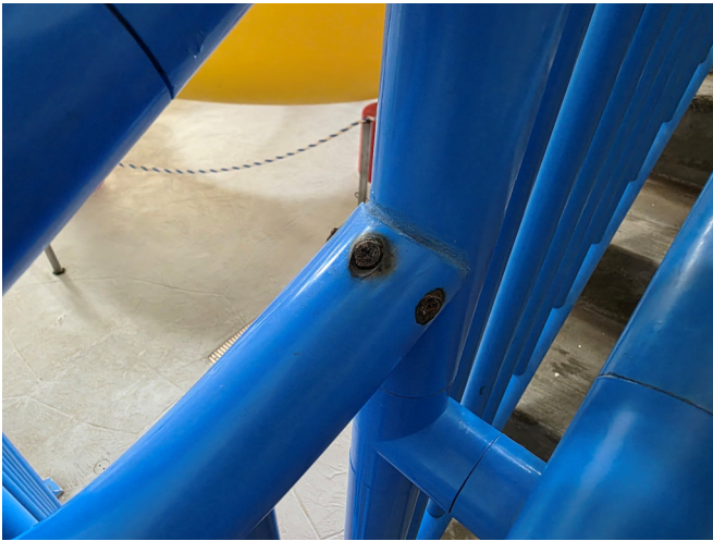
3. CORROSION ON FASTENERS
