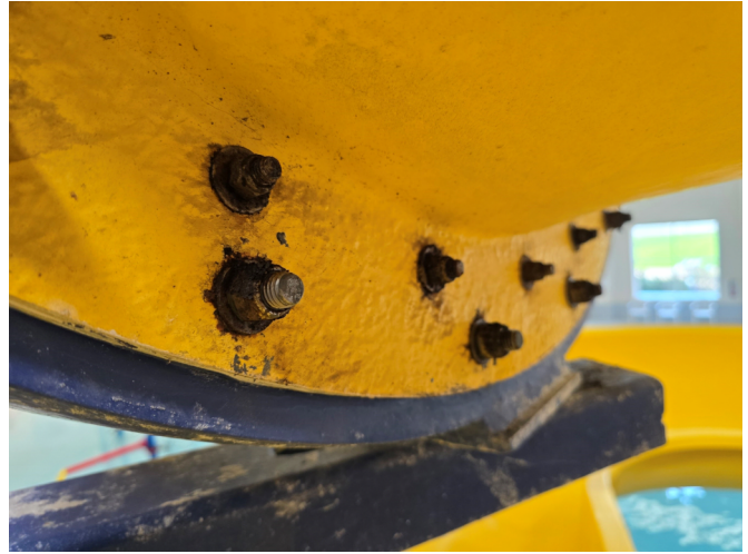
20. MISSING THREAD CAPS
