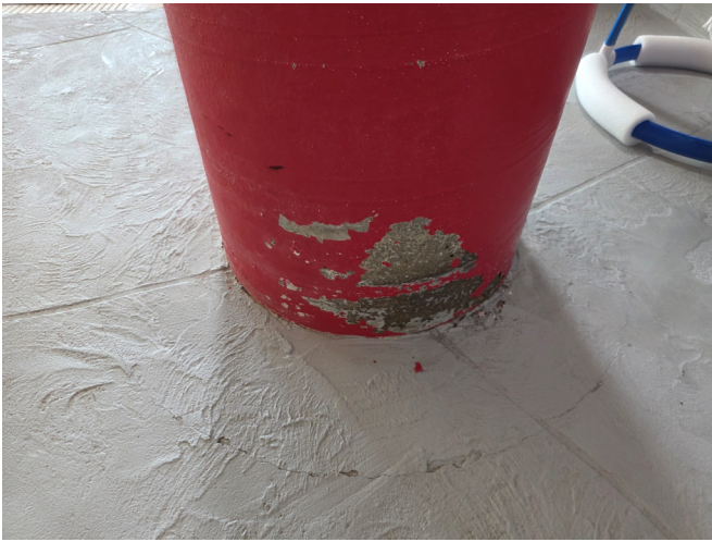
7. FLAKING/WORE PAINT AND FINISH
