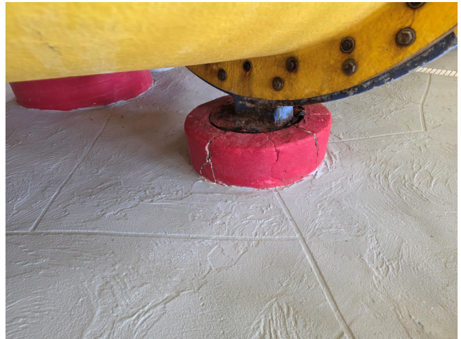
18. CRACKED PEDESTAL AND CORRODED SUPPORT PLATE
