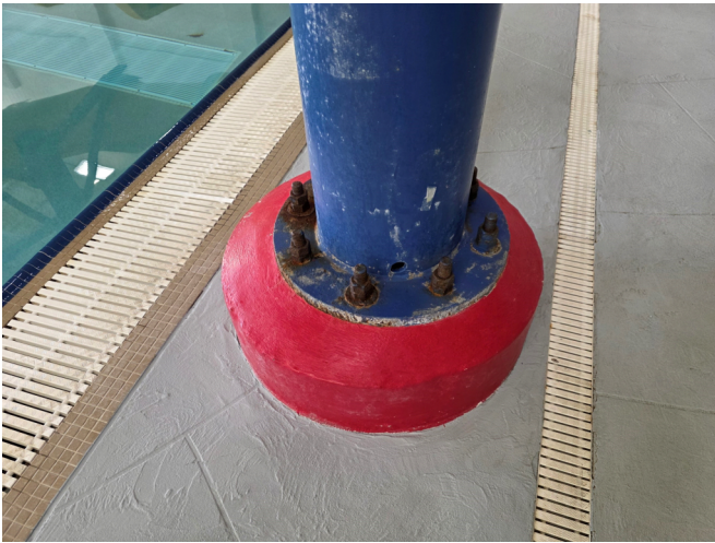
21. MISSING THREAD CAPS
