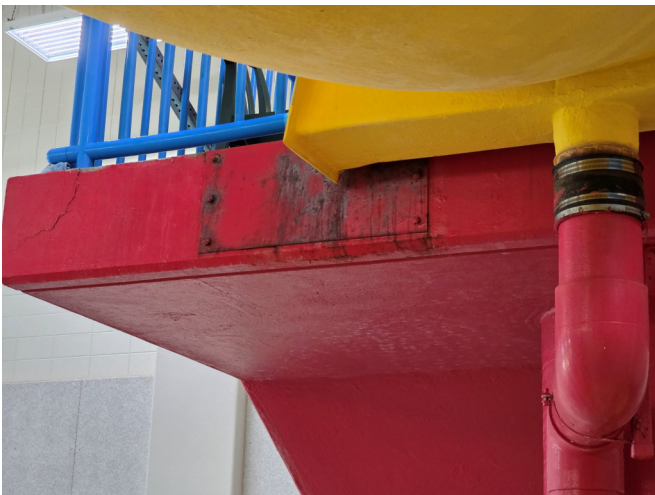
11. CORROSION ON METAL PLATE UNDER STARTING TUB
