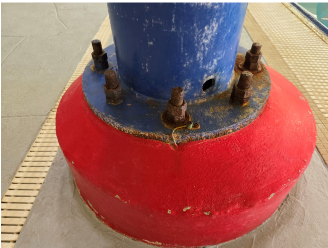
17. CORROSION ON SUPPORT TREE FLANGE AND FASTENERS
