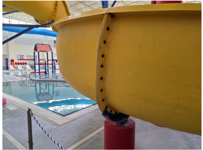
4. CORROSION ON FASTENERS
