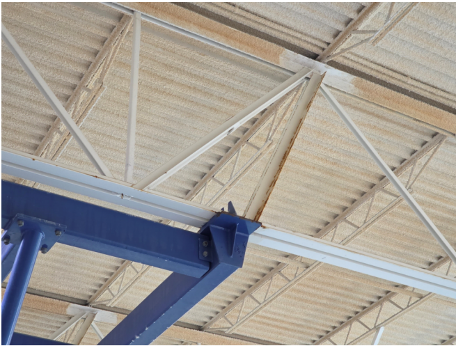
15. CORROSION ON ROOF/CEILING SYSTEM
