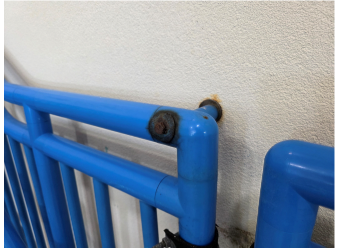
2. CORROSION ON FASTENERS
