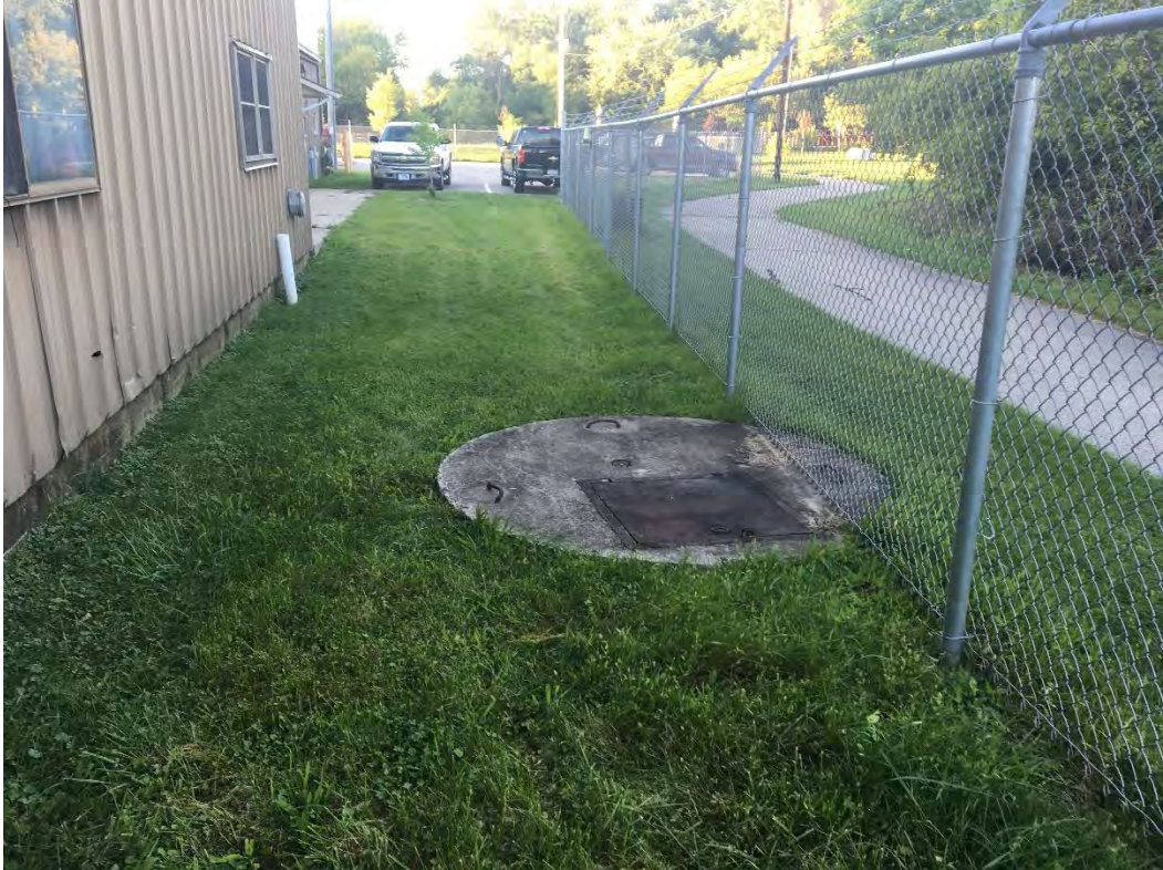
Looking South at storm sewer manhole upstream of outfall to Whitewater Creek
