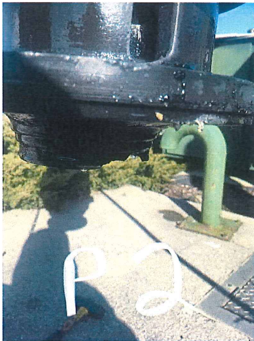
Figure 1 - Marketplace Lift Station Impeller Damage
