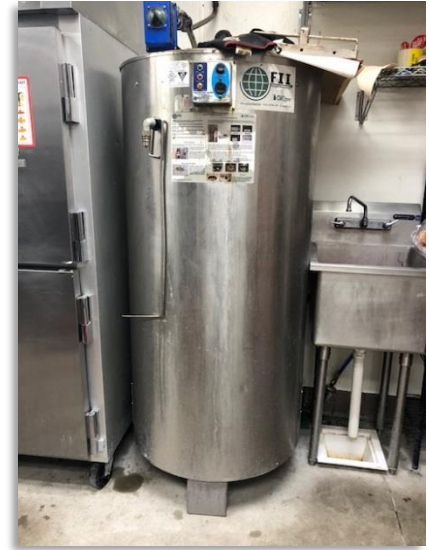
Grease Control Device at Sonic Restaurant
