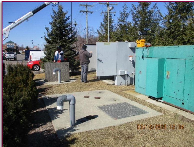
Village Lake Estates Pumping Station
