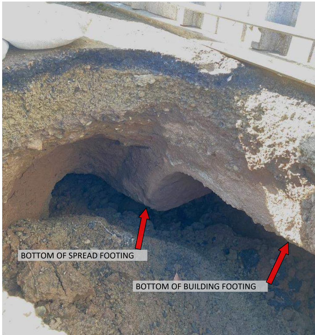
Photo 3: Exposed Foundation and Spread Footing, Tunnel to the Southeast of the Hole
