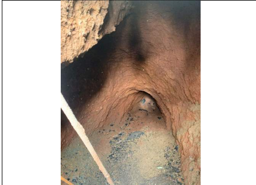
Looking North down void toward 4 th Street. Eastern perimeter footing is visible at top left corner of photo, and Brick structure is observed at end of void.
