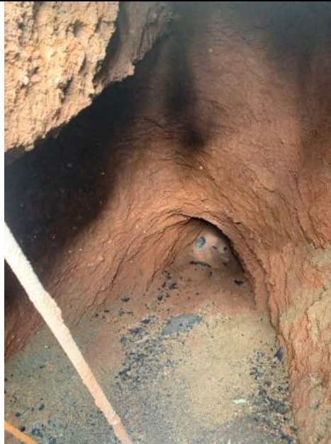
Looking North down void toward 4 th Street. Eastern perimeter footing is visible at top left corner of photo, and Brick structure is observed at end of void.
