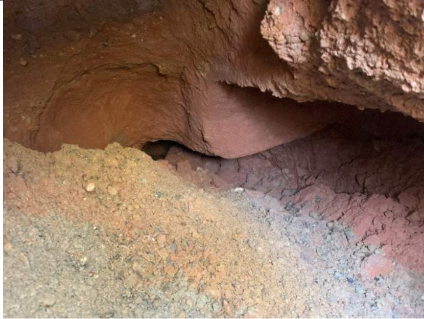
Looking Southwest below southeast corner of shop/warehouse building. Corner and eastern perimeter footing are visible.
