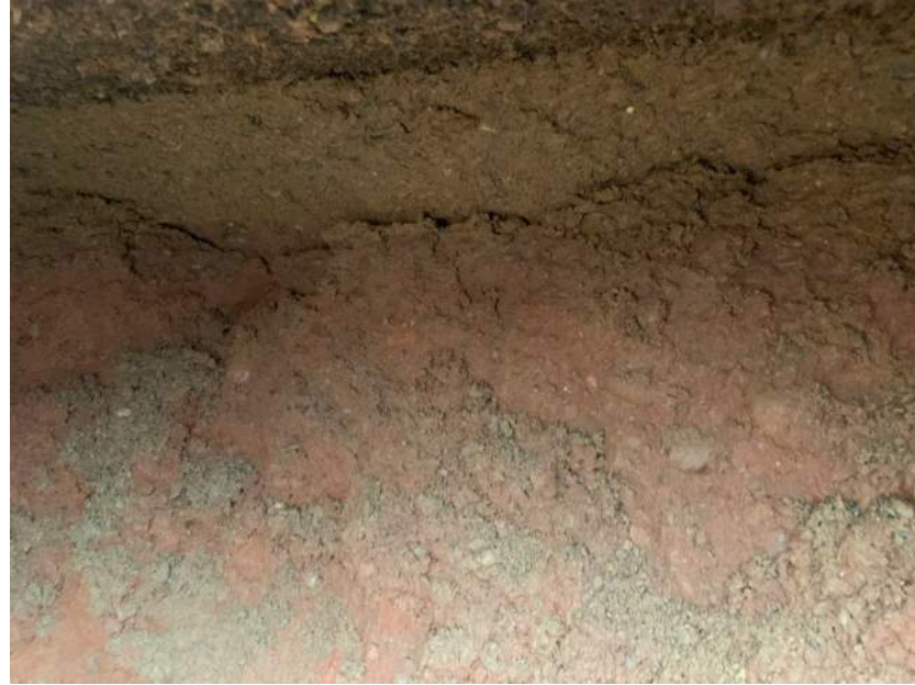
Undermined asphalt pavement at east edge of void. Bottom of AC is observed at top of photo.
