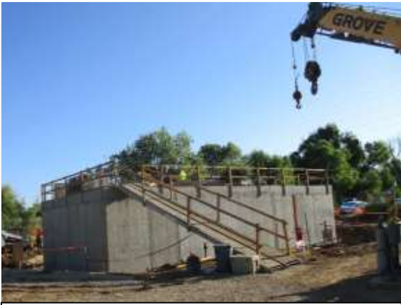
SRWA, Raw Water Pump Station, 2020
