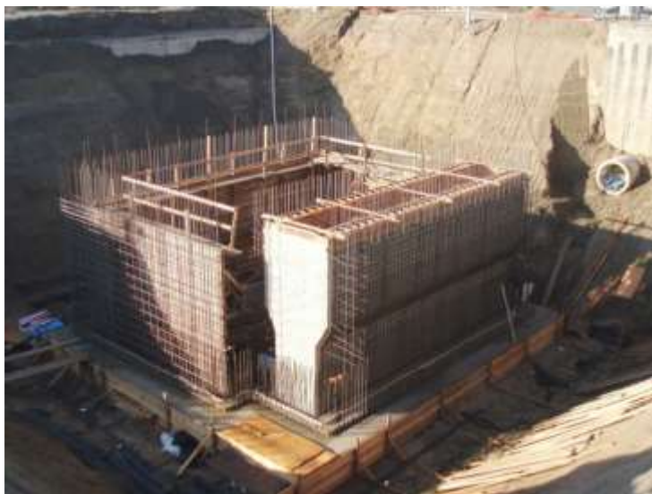
City of Manteca, Woodbridge Pump Station, 2008
