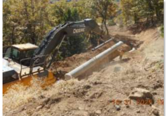
EID, Sly Park Intertie pipeline, current
