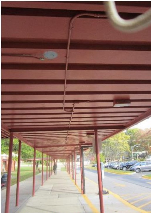
Exterior lighting in need of update & additional fixtures.
