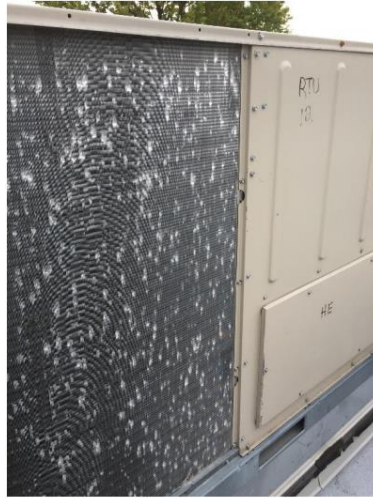
Damaged condenser coil fins.
