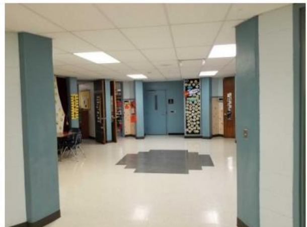
No egress at end of corridors
