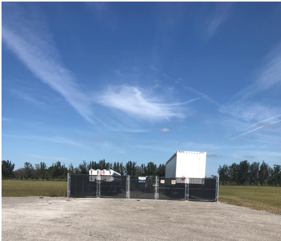
Existing Temporary Gas Utility Facility
