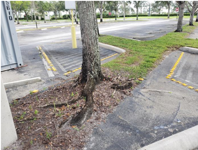
Example of 7" DBH Mahogany in narrow median with surface root damage to asphalt.
