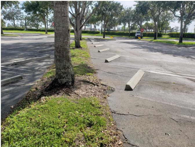
Example of 8" DBH Mahogany in very narrow median breaking up pavement.
