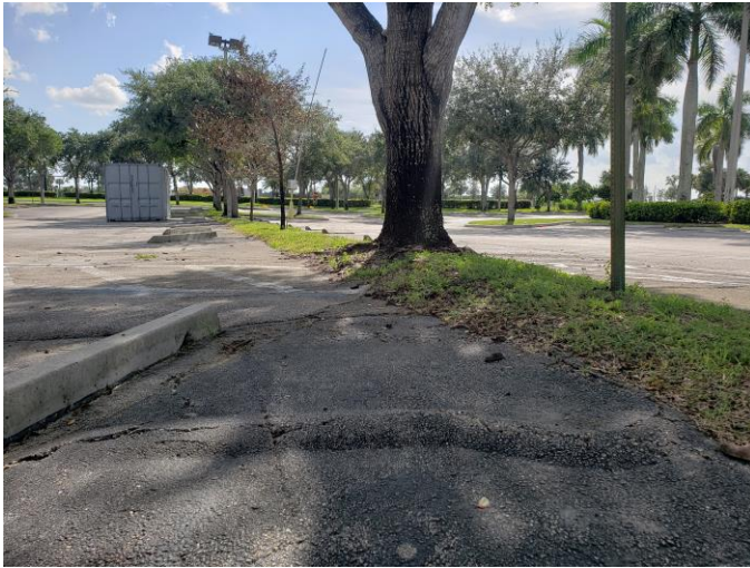
Example of 15" DBH Mahogany tree in median (proposed for removal) with co-dominant trunks. Note the root damage.
