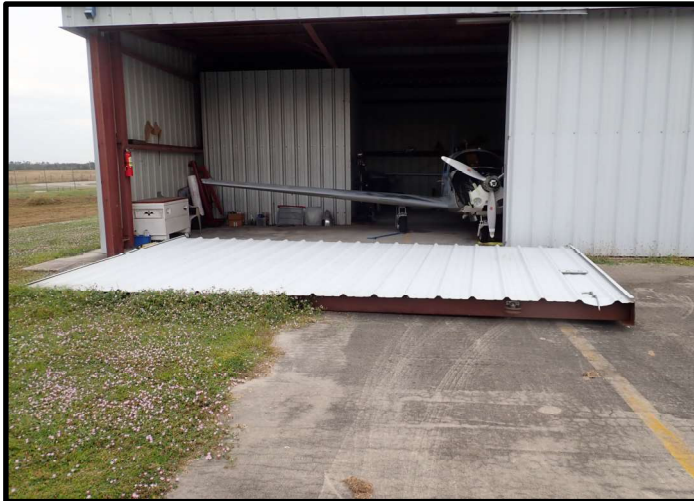
Photograph 3 - Damaged steel framed door.
