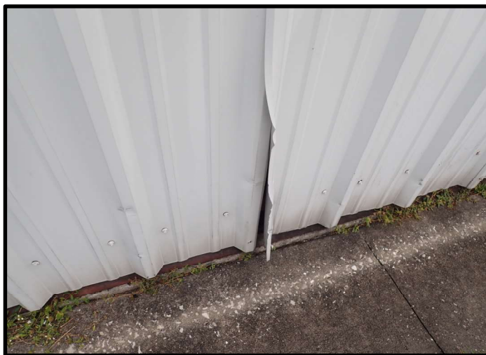
Photograph 4 - Pre-existing damage at metal wall panel.
