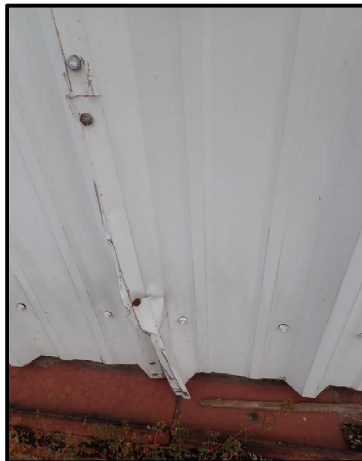
Photograph 2 - Pre-existing damage at metal wall panel.
