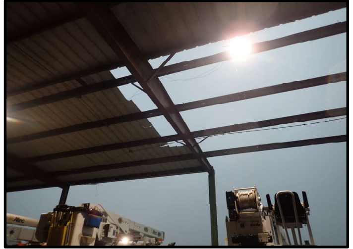
Photograph 2 - Missing roof panels.
