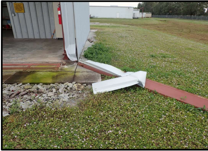
Photograph 5 - Steel column damage.
