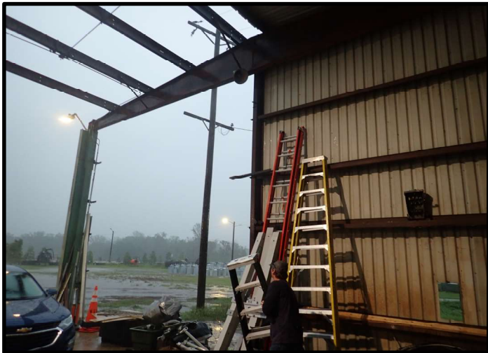
Photograph 3 - Missing roof and wall panels.
