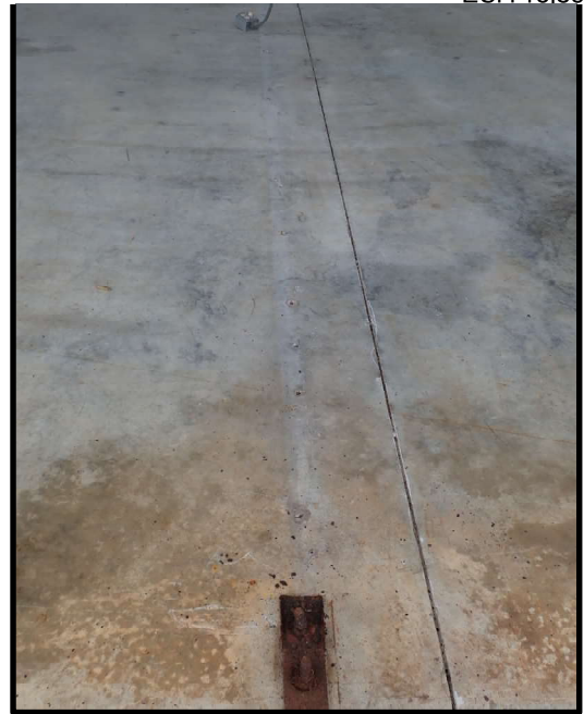
Photograph 6 - Location of detached demising wall bottom track.
