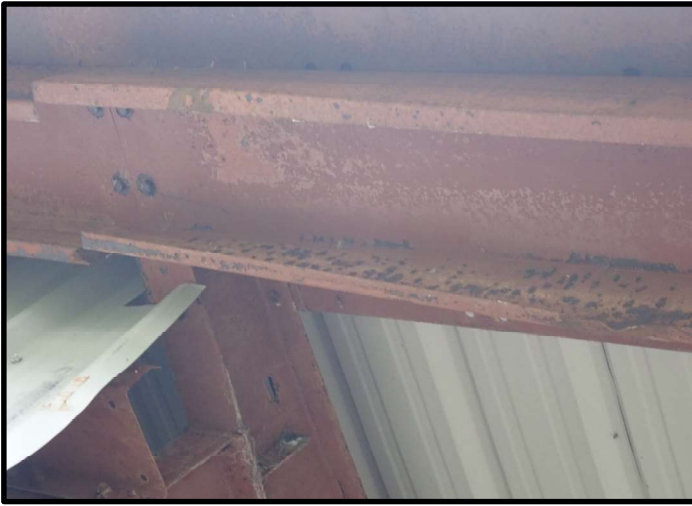
Photograph 5 - Damaged steel door track.
