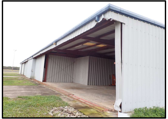
Photograph 6 - Location of (2) missing doors.
