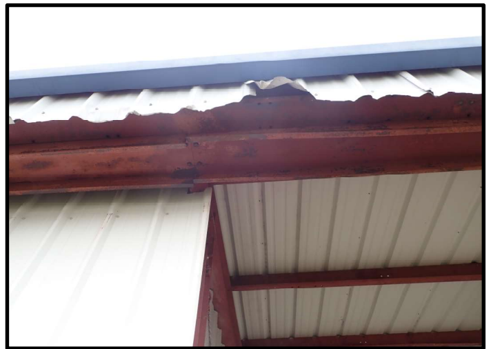
Photograph 4 - Metal wall panel and steel door track damage at roof.
