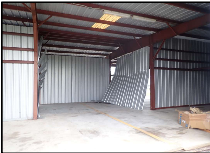
Photograph 3 - Damaged wall paneling.
