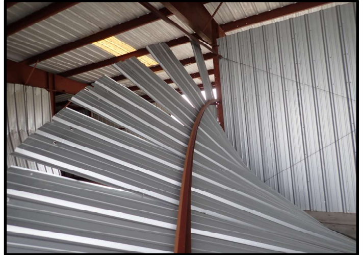
Photograph 2 - Damaged girt and wall paneling.
