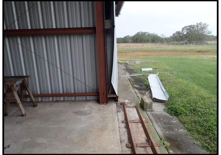
Photograph 2 - Damaged wall panel.
