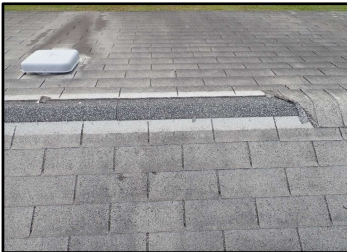
Photograph 3 - Closeup of ridge shingles missing.
