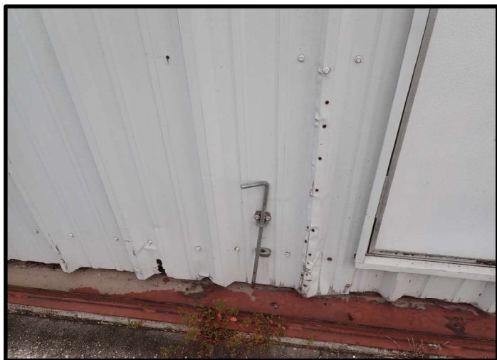
Photograph 3 - Pre-existing damage at metal wall panel.
