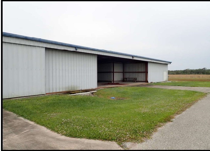
Photograph 1 - Overall view of hangar exterior with missing doors.
