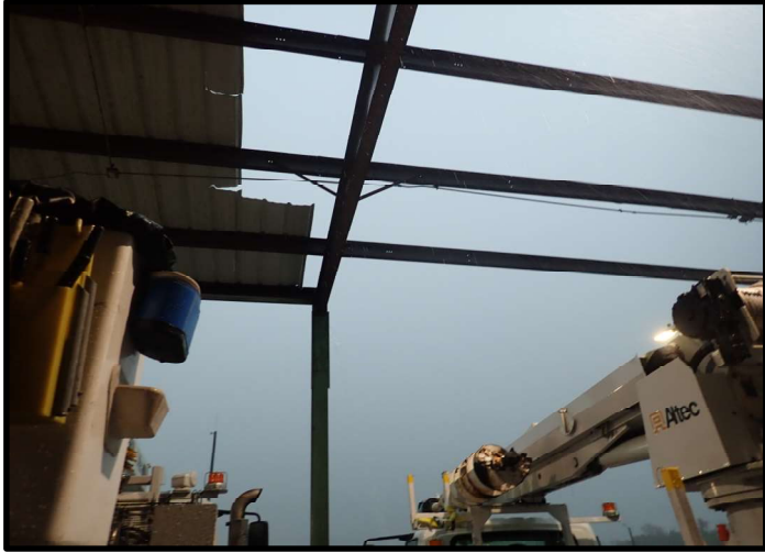
Photograph 1 - Missing roof panels.
