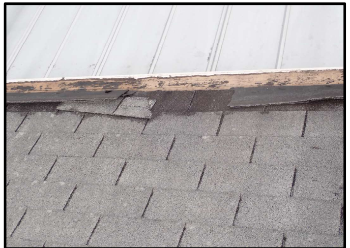
Photograph 4 - Closeup of shingle starter course missing.
