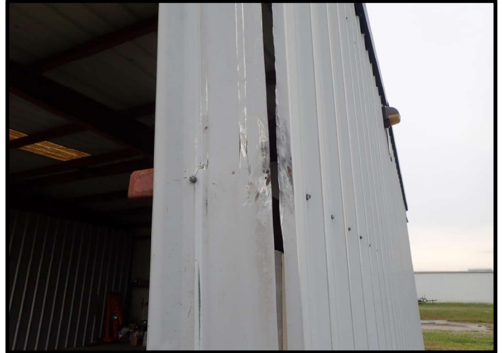
Photograph 2 - Metal wall panel damage.
