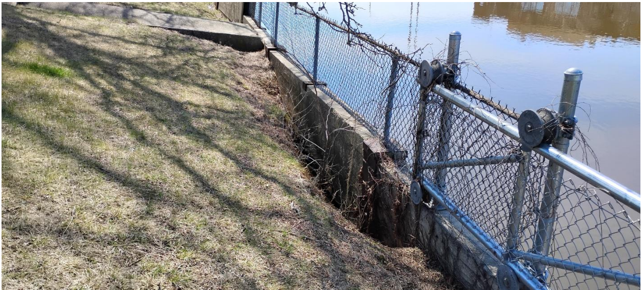
Figure 5. Lost fill in Section C. Surface drain from parking lot seen near top of photo.
