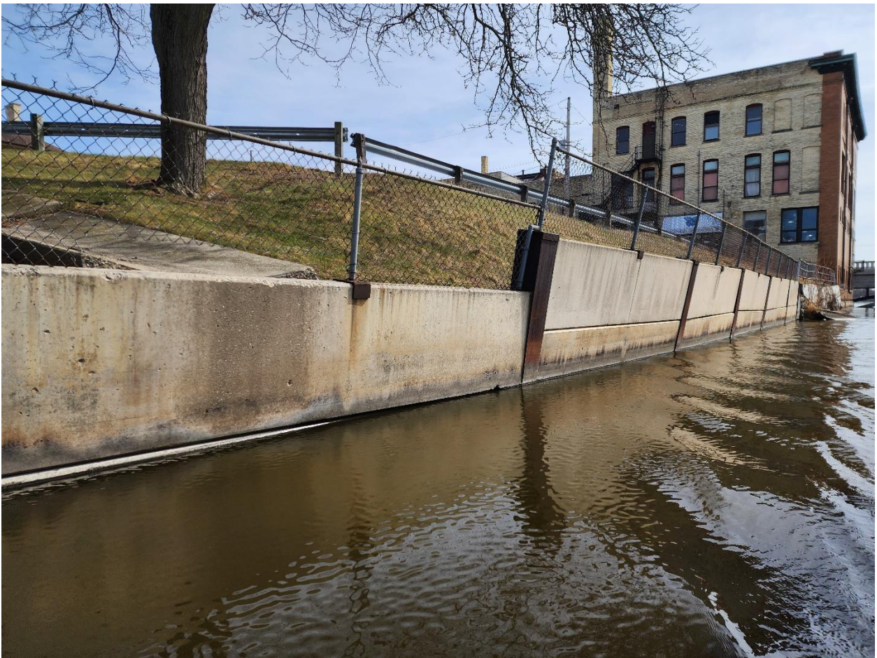
Figure 4. View of extreme deflection in Section B.
