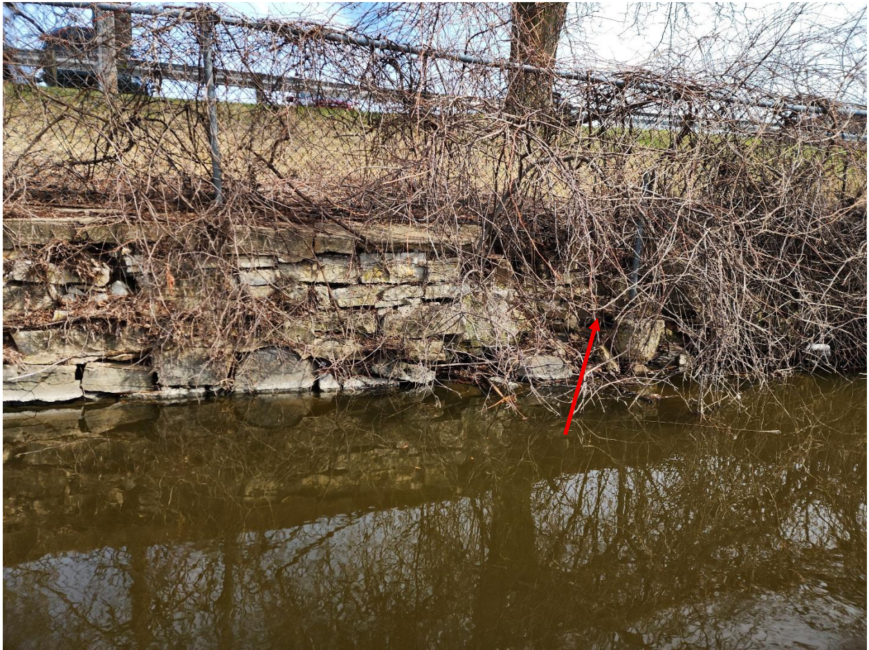
Figure 6. Failed portion of Section D.
