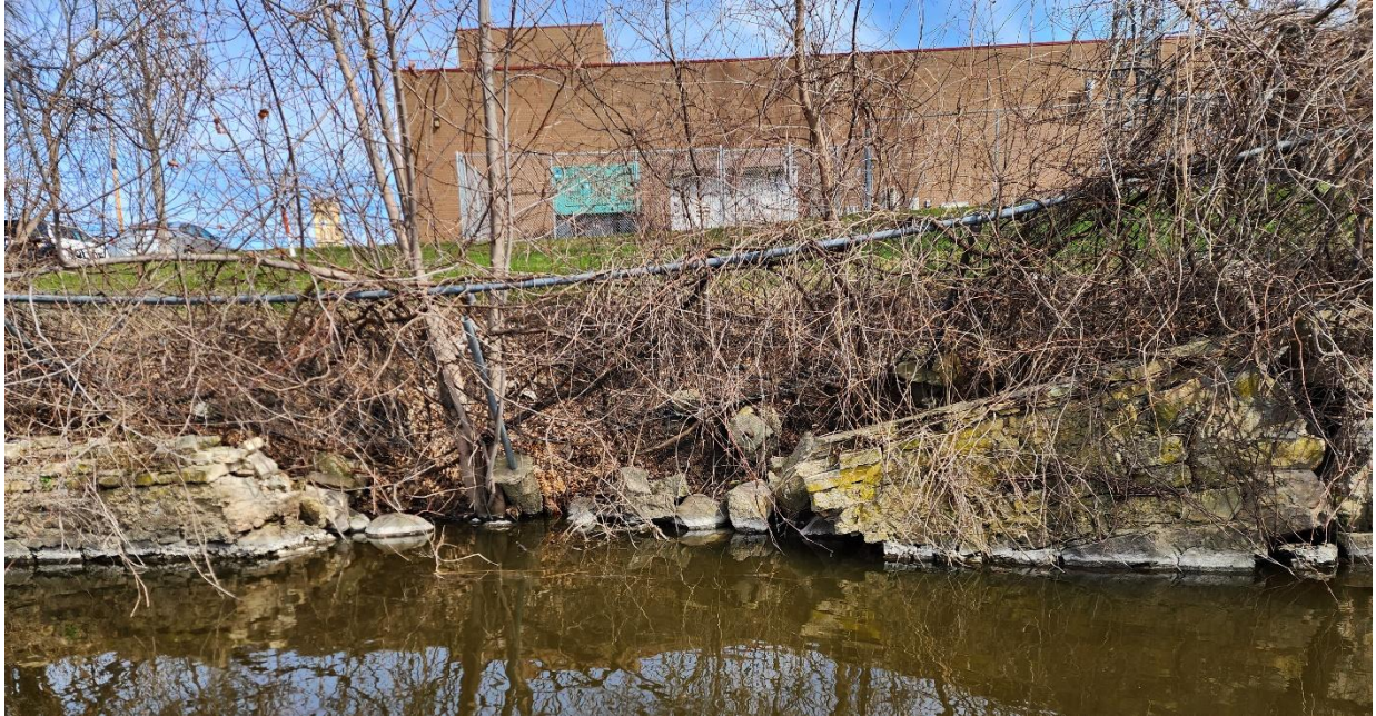
Figure 7. Failed segment of wall along Section E.
