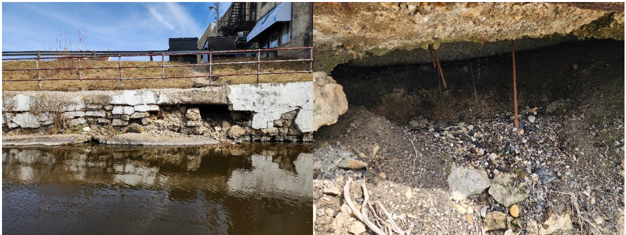
Figure 3. Location of void below surface drain (left) and depth of void (right).
