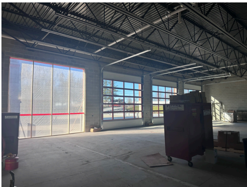
The apparatus bay doors went in. The first floor framing is mostly done.
