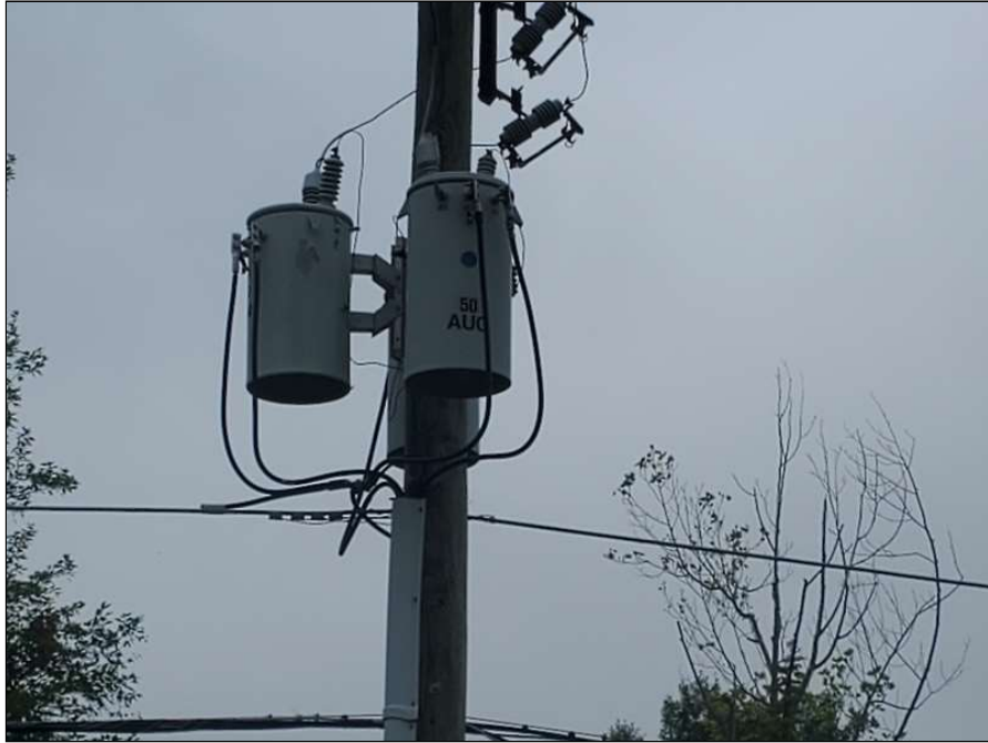
3 - Non-pcb transformers on northwestern portion of site
