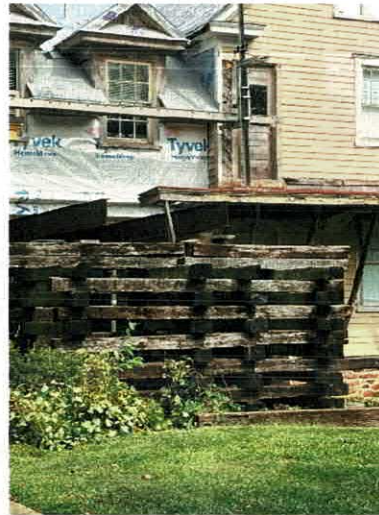
(Picture 5: Shows faulty structural supports, inadequate roofing, and exposure to the elements)
