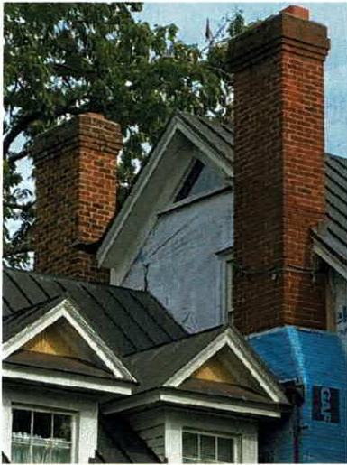
(Picture 7: Shows inadequate protection From the elements)
