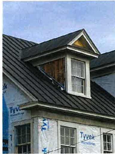
(Picture 8: Shows inadequate roof drainage, and inadequate protection from the elements)
