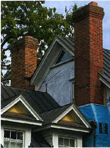
(Picture 7: Shows inadequate protection From the elements)
