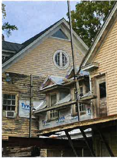
(Picture 2: Shows faulty structural supports, inadequate roofing and exposure to the elements)
