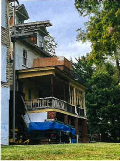
(Picture 12: Shows inadequate protection From elements and inadequate Structural supports on porch)
