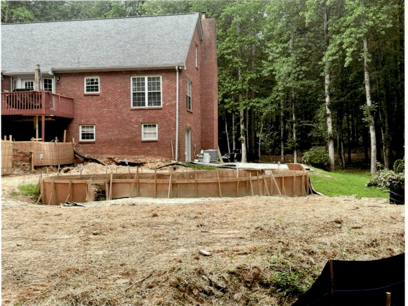
View from the back side of the pool area showing framed pool and location relative to the home.
