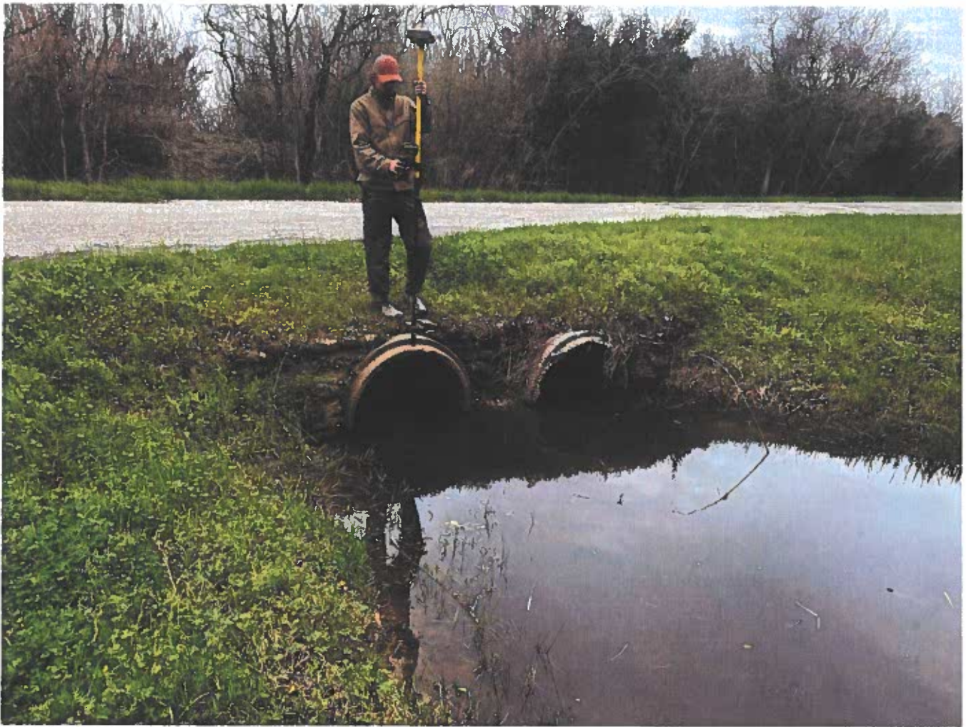
Figure 4. View of culverts on the east side of Penick Road. The culvert on the right is blocked and inactive. The culvert on the left is actively flowing. The water surface observed in this photo was measured at 182.5 feet elevation.
