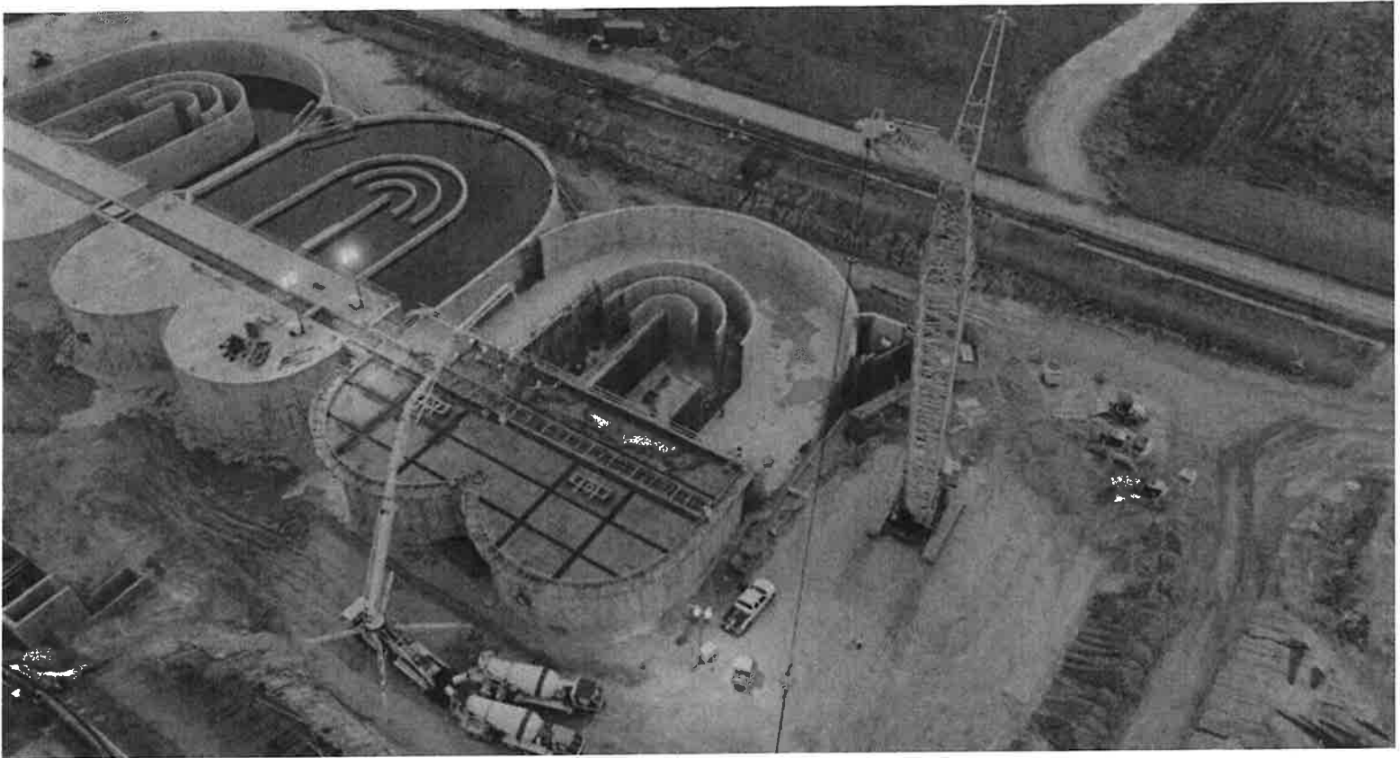
▲ Horse Creek Pollution Control Facility
