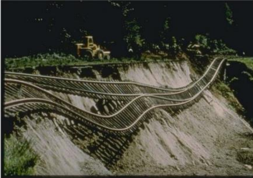
Figure 3: During the 1965 Puget Sound Earthquake, a large portion of the railroad lines north of the old brewhouse were significantly damaged in an earthquake induced landslide.
