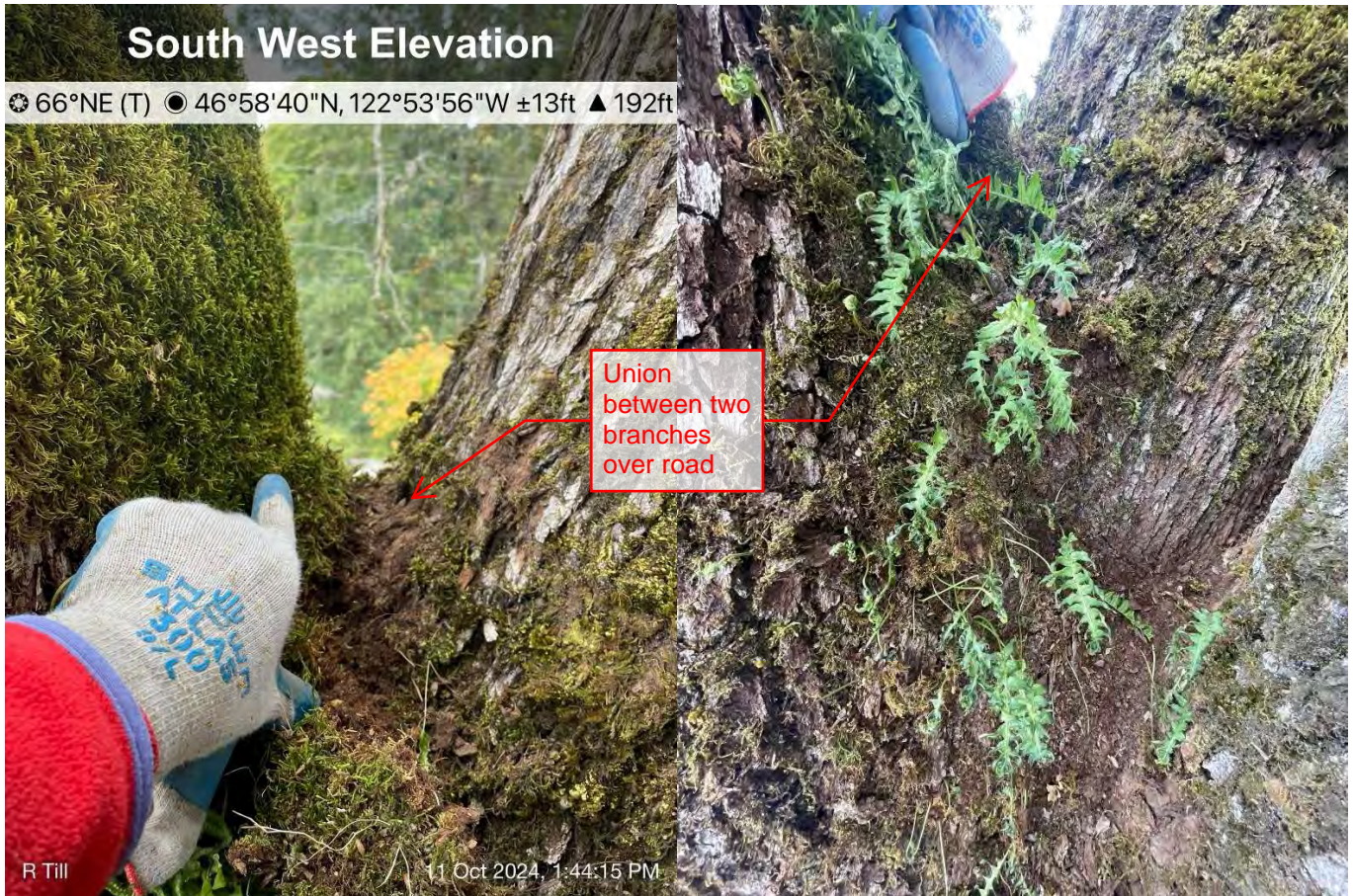
Figures 7 and 8 Southwest view of attachment between two secondary stems extending over the road. Exterior signs indicate a sound union.
