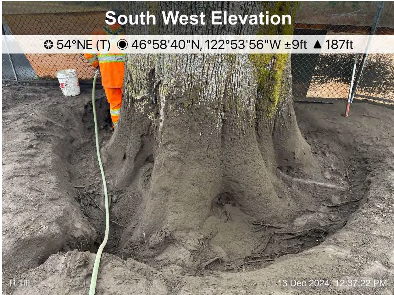
Figure 3 Full view of excavation from southwest. All visible portions were inspected and no indicators of decay identified.
