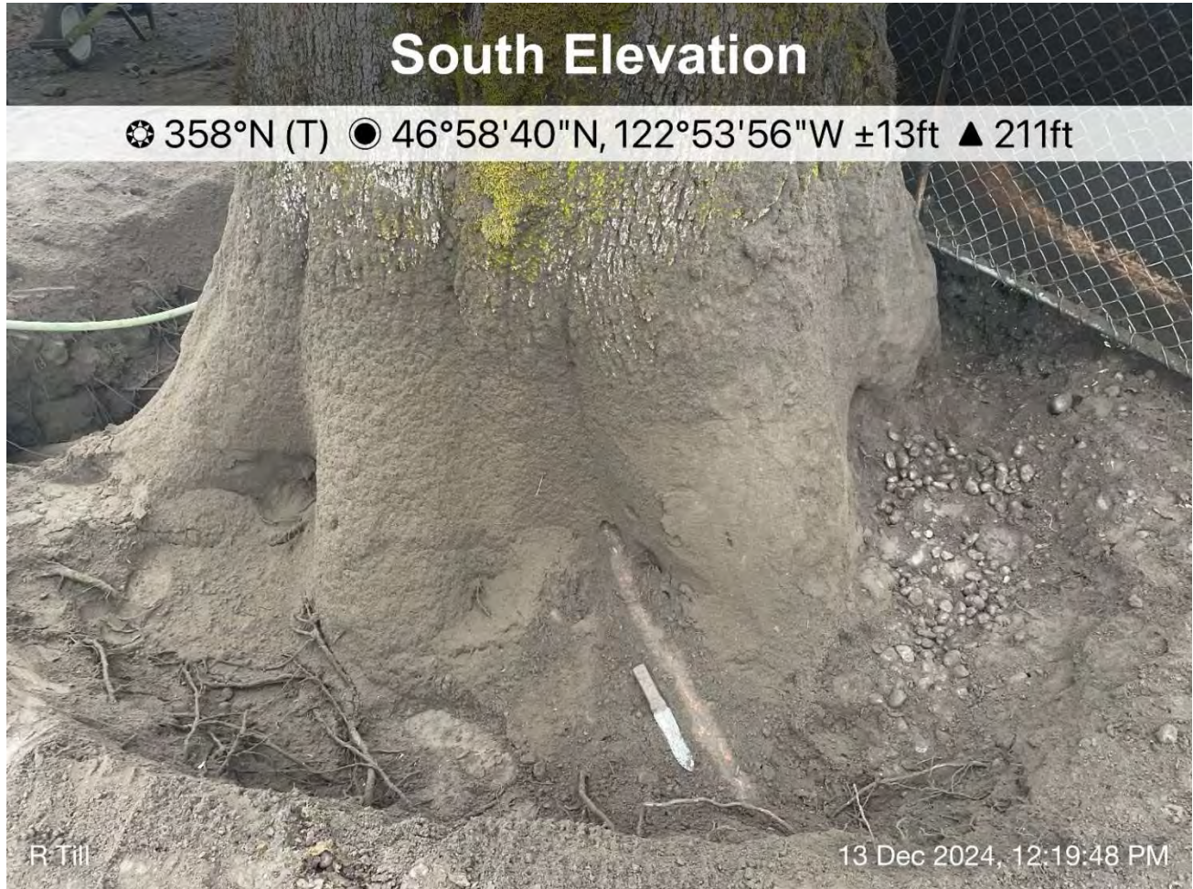
Figure 2 Southeast side excavated to significant lateral root. Performed additional probing to locate solid buttress roots and solid integrity of wood between buttress roots.
