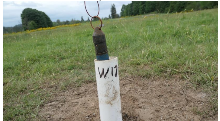
Photo 76. Datalogger installed within monitoring wells
