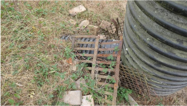
Photo 69. Ditch drains to this make-shift catch basin
