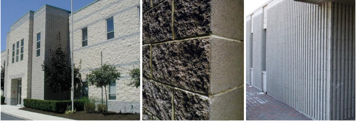
Figure 5.D.5-5. Acceptable concrete block textures, including a mixture of split-faced concrete block and smooth-faced concrete block (left and middle examples) and fluted or grooved concrete block (right example).
