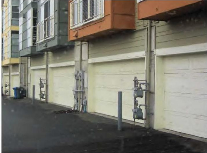
Figure 2.B.6.1-3. Place utility meters in less visible locations. Note that this example is acceptable on a service alley but not near a street or residential walkway.
