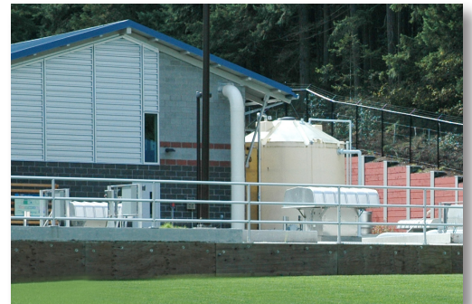
Martin Way Reclaimed Water Plant
