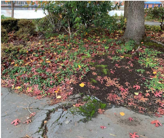
HEAVING / CRACKING PAVING
