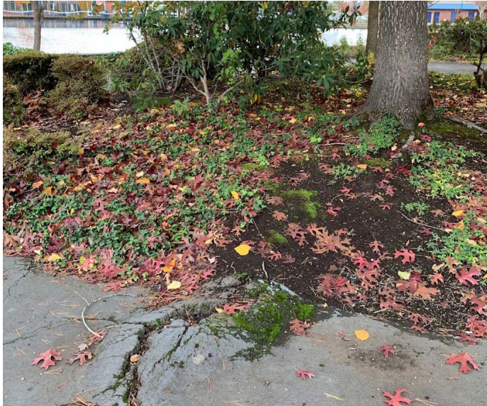
HEAVING / CRACKING PAVING
