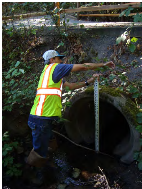
Site location: Culvert crossing under trail Photo number: H3-22 Description: Looking downstream, confluence with tributary from the south
