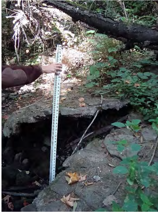
Site location: 200' upstream of Tualatin River Photo number: H1-5 Description: Concrete poured in channel from left bank
