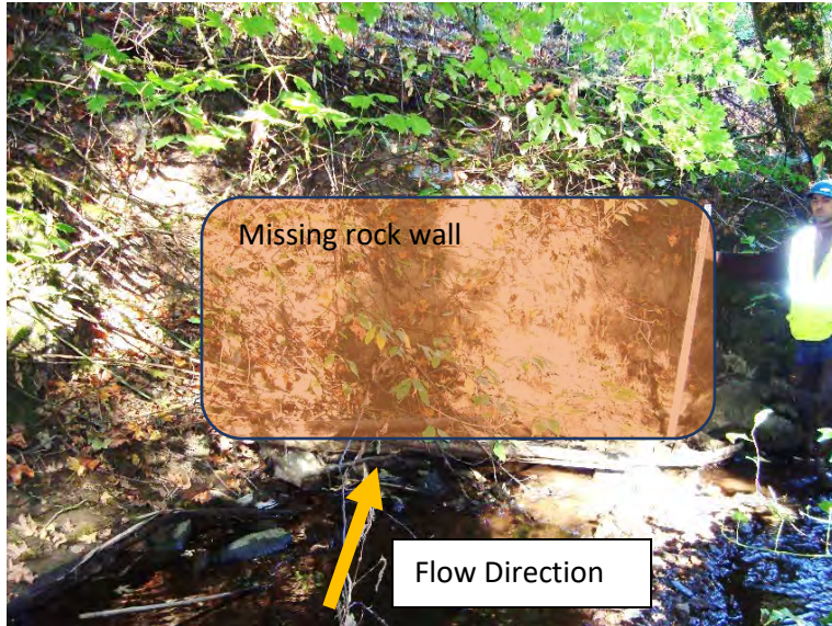
Photo 11. Hedges Creek Reach #3A, showing rock wall location and missing rocks.
