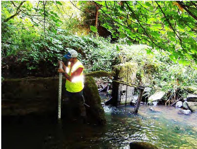
Site location: ~850' upstream of Tualatin, 20' upstream of culvert Photo number: S1-7 Description: Old 3' high concrete weir wall (2 ½' wide opening) with pool on downstream end. Weir is leaning downstream and sediment has deposited behind it on upstream side.
