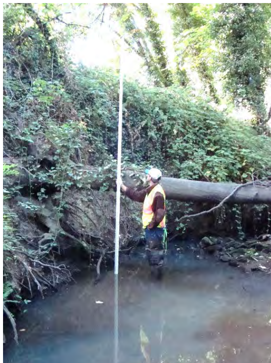
Site location: 150' upstream of Tualatin River Photo number: H1-4 Description: Looking upstream, right bank erosion, downed trees, slumping on right bank
