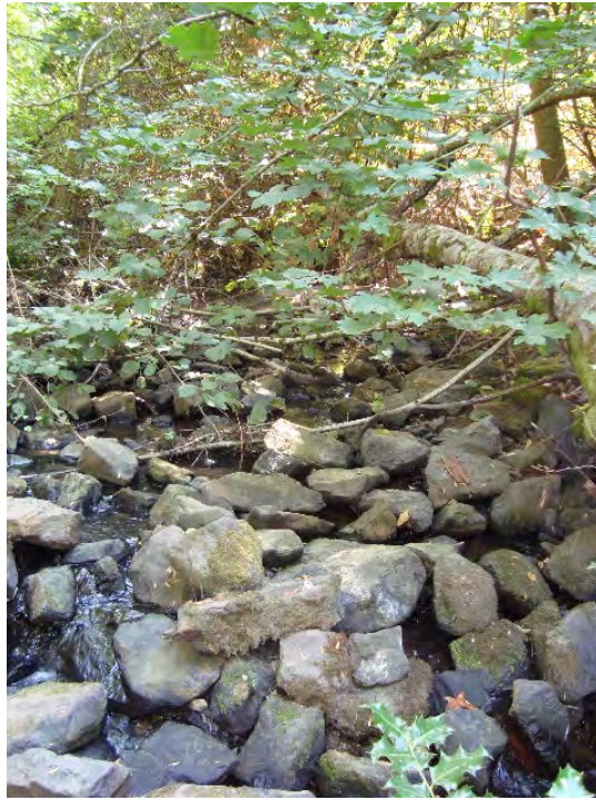
Site location: Immediately downstream from confluence with S. tributary Photo number: H3-21 Description: Looking upstream, riprap
