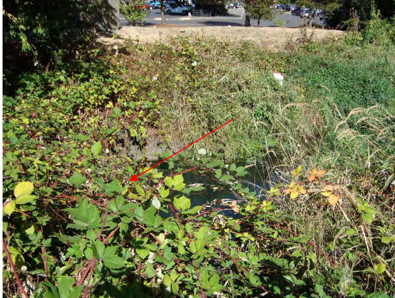
Site location: East side of SW SW Martinazzi Ave. Photo number: N3-1 Description: Looking downstream of SW Martinazzi Ave. where 48-inch diameter stormwater pipe enters Nyberg Creek (approximately where red arrow is pointing)
