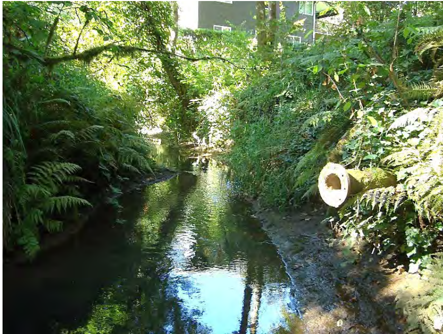
Site location: 600' upstream of SW Borland Rd. Photo number: S1-21 Description: Broken pipe (right side of photo) on left bank, looking upstream
