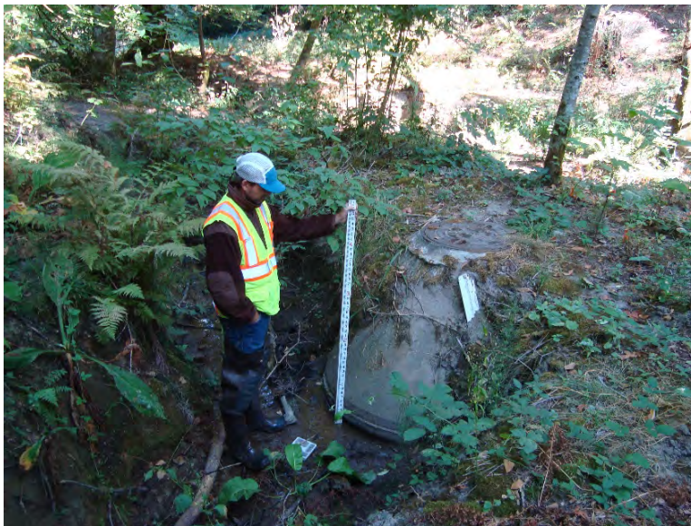
Photo 12. Side channel incision and erosion around sanitary sewer manhole.
