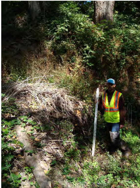
Site location: 1100' upstream of SW 105 th Ave. Photo number: H3-16 Description: Right bank slope failure, very wet
