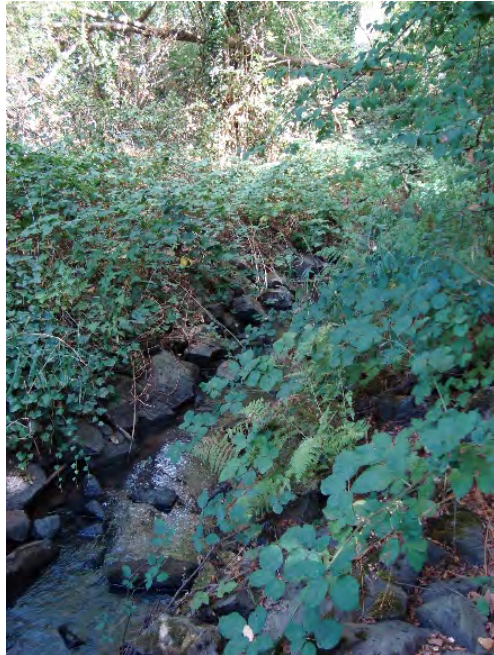
Site location: Culvert at SW Tualatin-Sherwood Road Photo number: H2-1 Description: Armored channel with rip-rap, looking downstream
