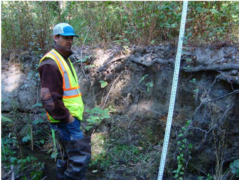
Site location: 900' upstream of SW 105 th Ave. Photo number: H3-14 Description: Outside bend erosion
