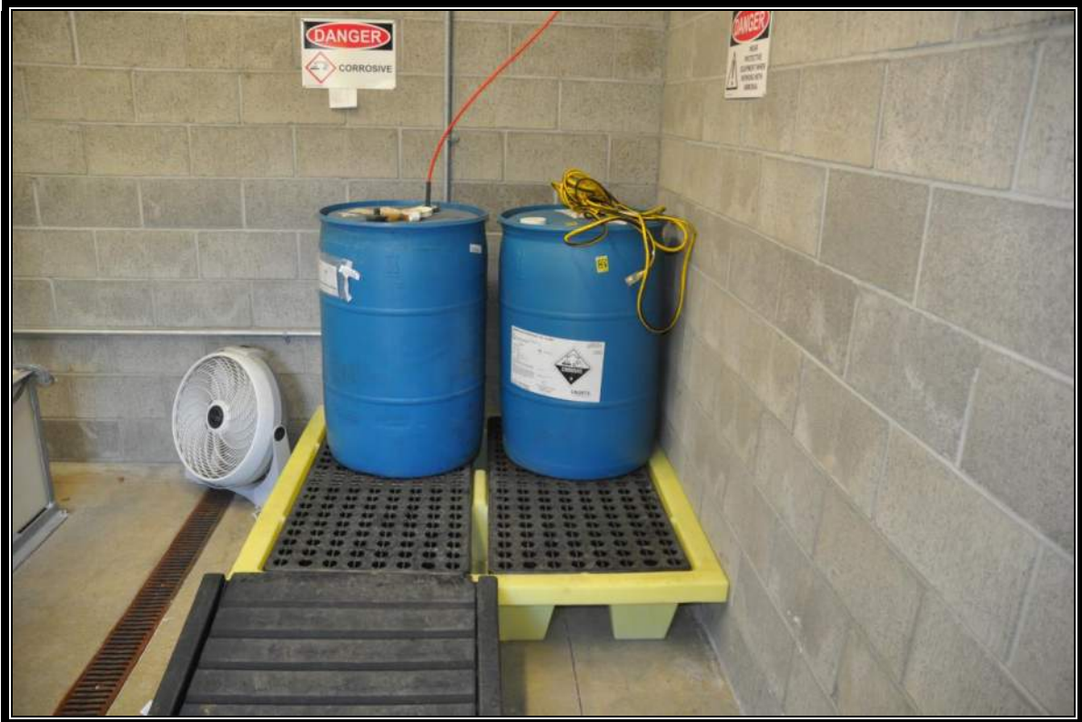
ASR Pump Station – Unbraced Chemical Barrels
