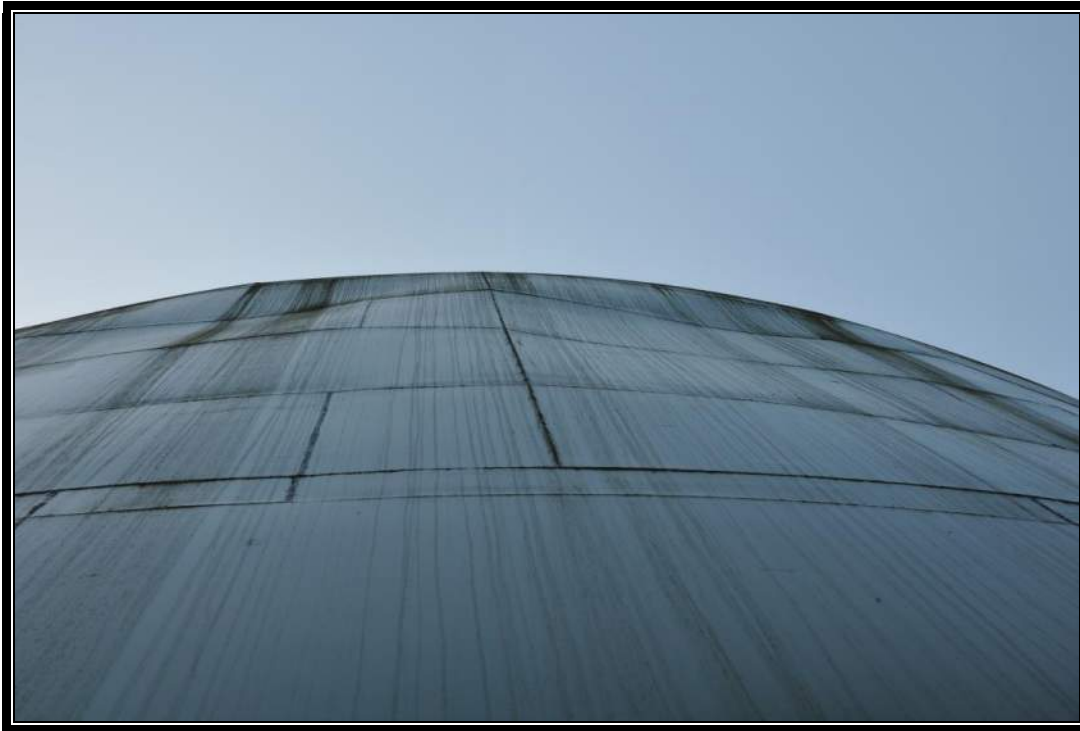
2.2 MG B1 Reservoir – Wall Shell Plate Buckling
