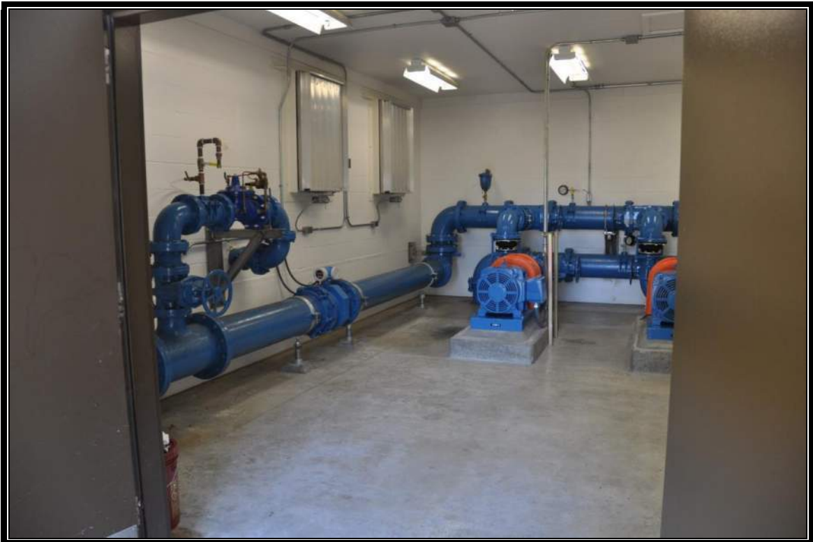
C Level Norwood Pump Station – Vertical Pipe Bracing, Limited Lateral Support
