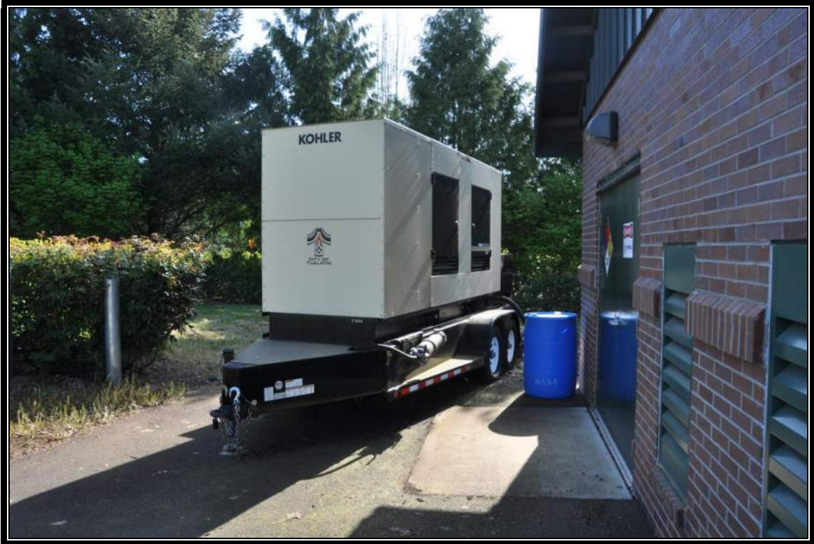
ASR Pump Station – Temporary Generator
