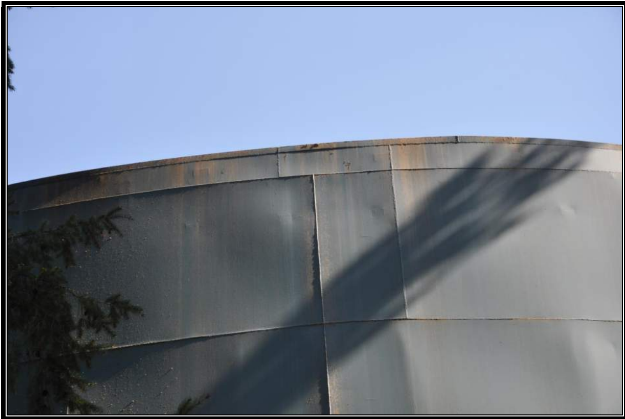
2.2 MG A1 Reservoir – Buckled Wall Shell Plates
