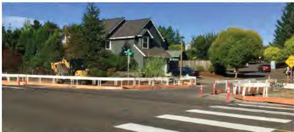
Construction is nearing completion at the new pedestrian crossing at Boones Ferry Rd and Siletz Dr in Tualatin
