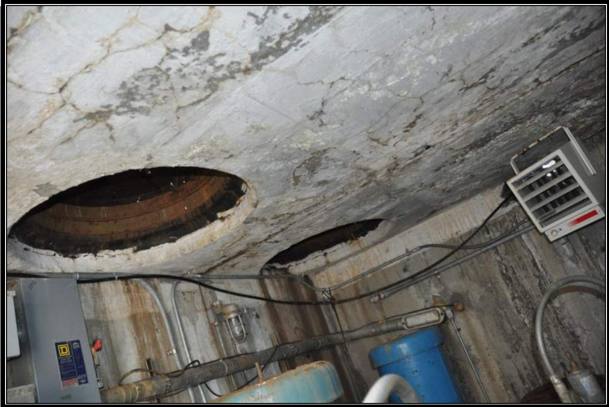
Martinazzi Pump Station – Bottom of Roof Panels Showing Poor Concrete Condition
