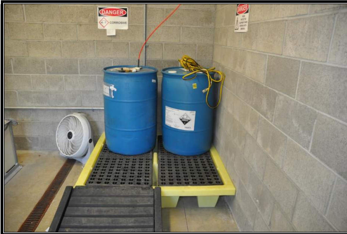
ASR Pump Station – Unbraced Chemical Barrels
