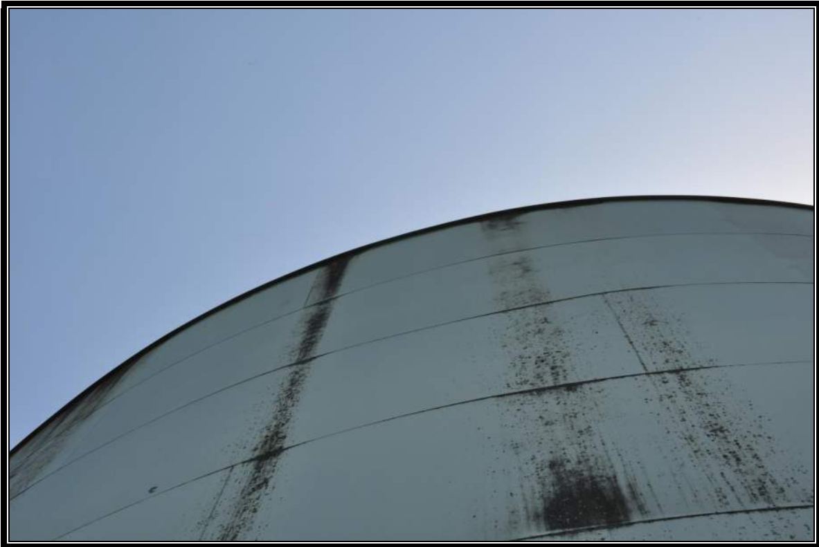
2.2 MG B2 Reservoir – Wall Shell Plates
