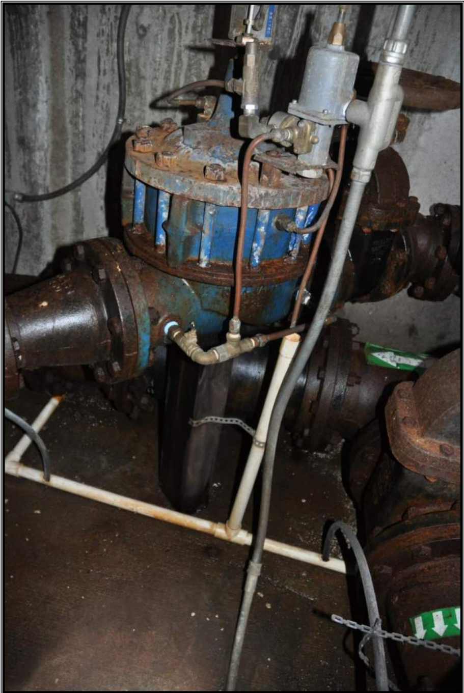
Martinazzi Pump Station – Outdated Pipe Bracing
