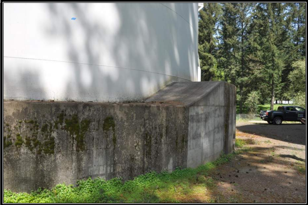
0.8 MG C1 Reservoir – Ballast Ring
