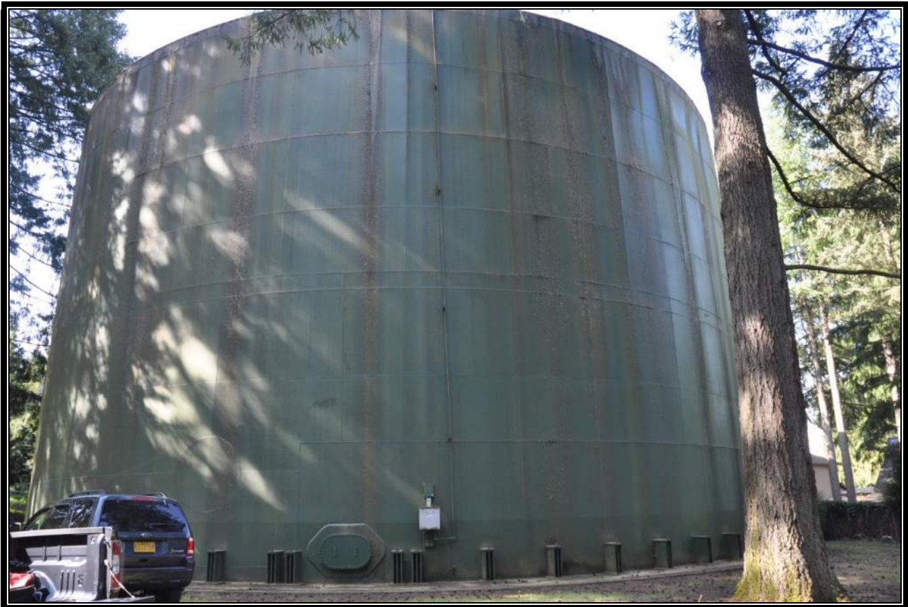
2.2 MG A1 Reservoir
