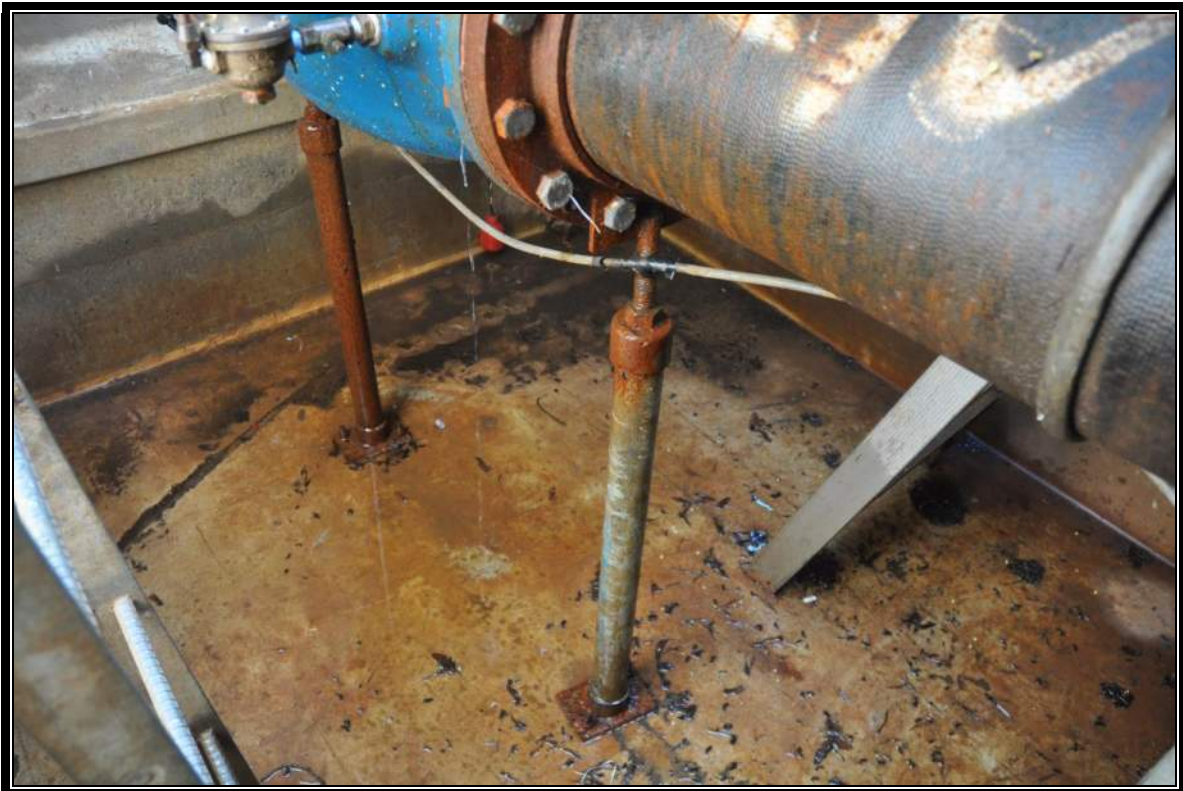
Boones Ferry Control Station – Vertical Pipe Bracing Only, No Lateral Bracing
