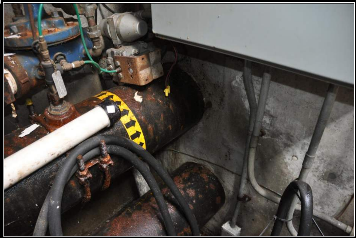
Martinazzi Pump Station – Rigid Pipe Penetrations Through Vault Wall
