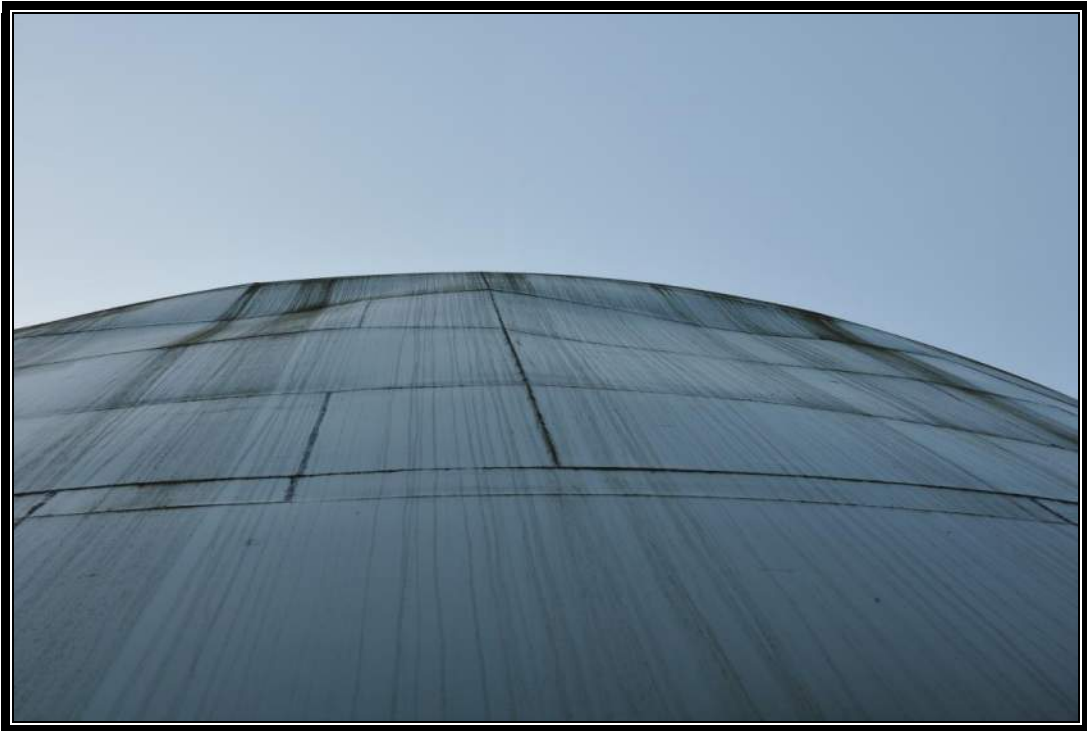
2.2 MG B1 Reservoir – Wall Shell Plate Buckling
