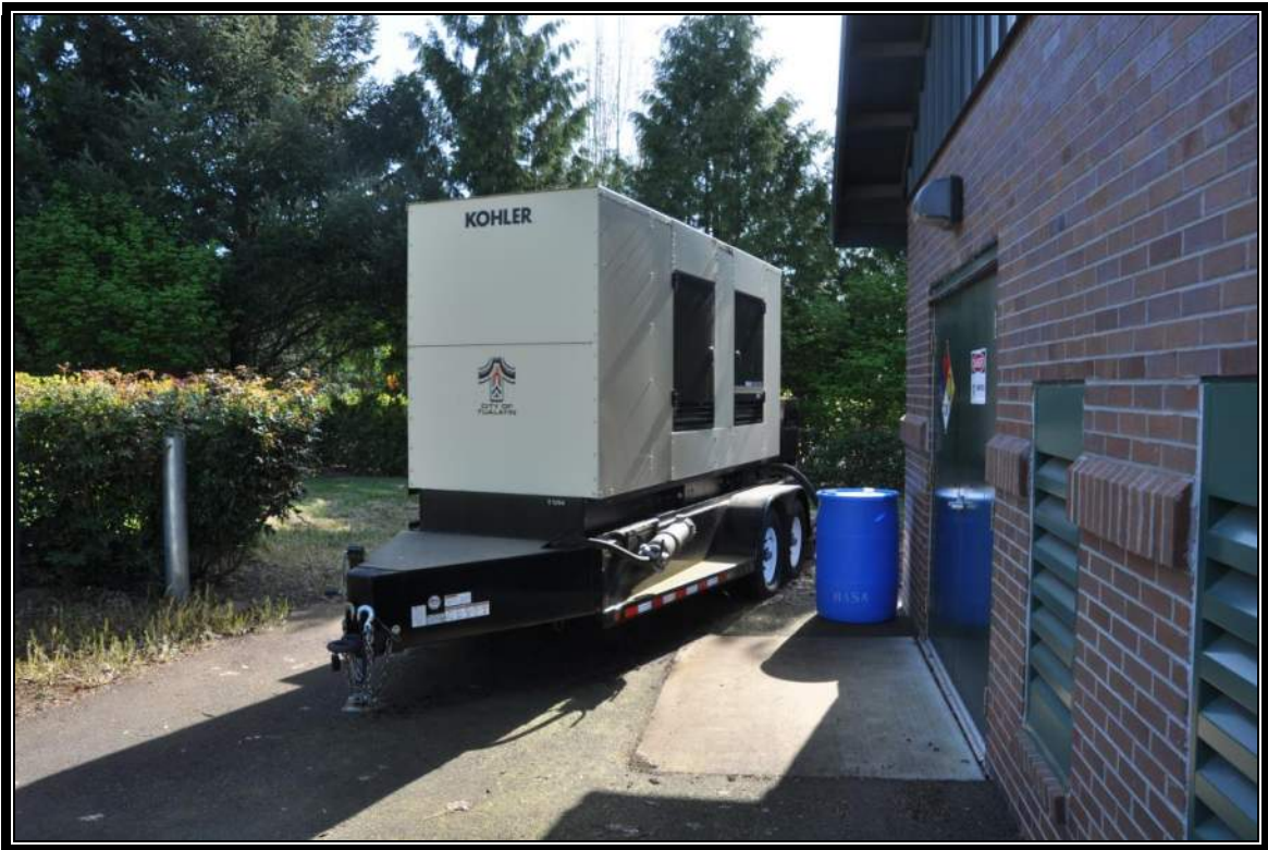
ASR Pump Station – Temporary Generator
