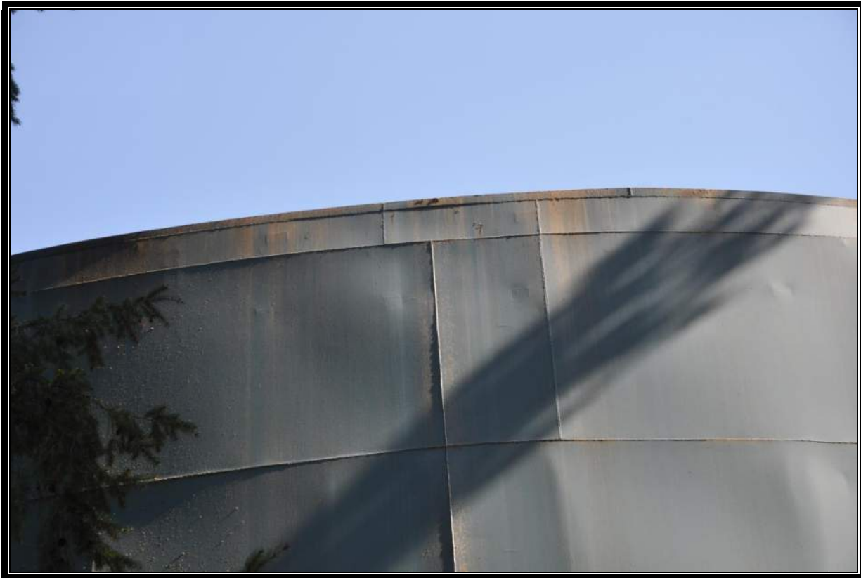
2.2 MG A1 Reservoir – Buckled Wall Shell Plates
