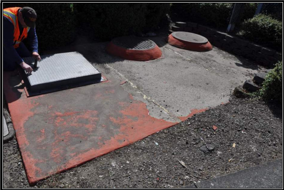
Martinazzi Pump Station
