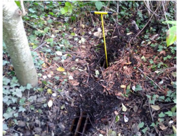
Figure 6-1. Example of buried outlet control structure at the Green Lot Swale
