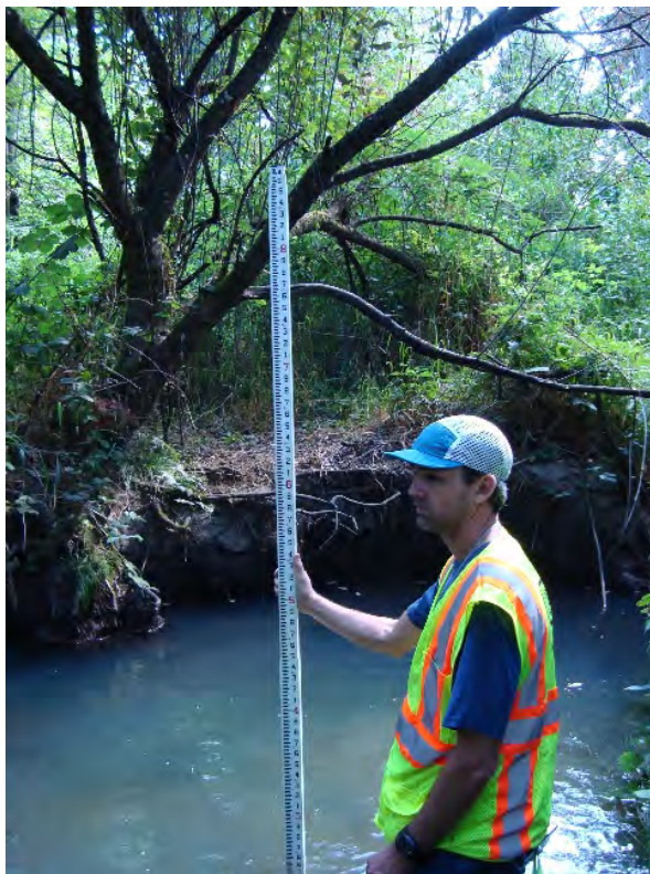
Site location: 600' upstream of SW Tualatin-Sherwood Road Photo number: H2-6 Description: Erosion on outside bend (right bank)
