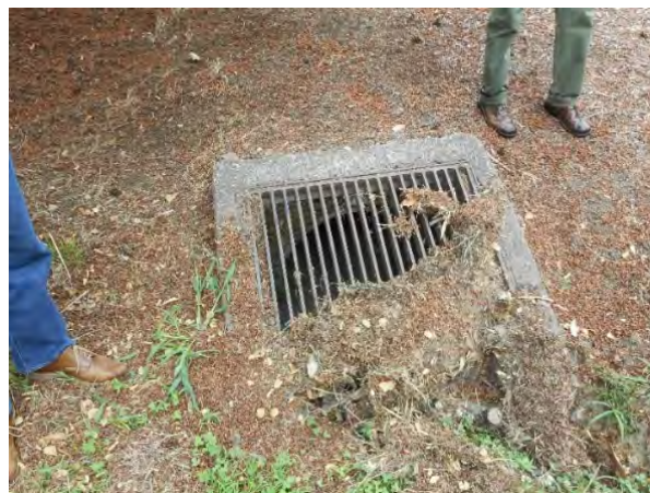
Image 2. Tree debris clogging the ditch inlet at the downstream end of the open channel
