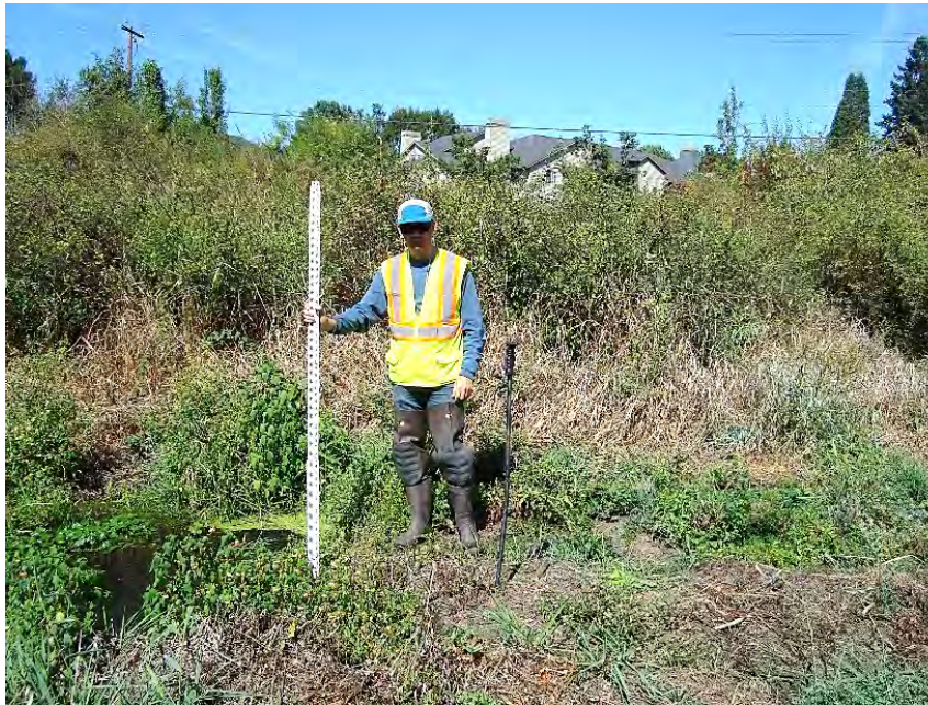
Site location: 200' upstream from SW Nyberg Lane Photo number: N1-4 Description: Old roadbed. Stream is in 30" CMP culvert under road.
