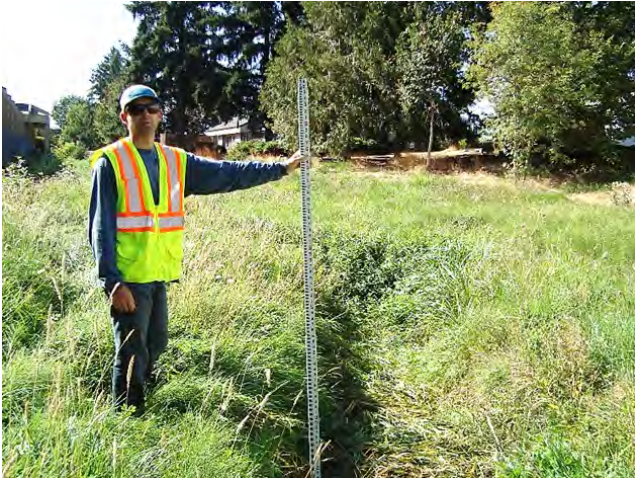
Nyberg Creek between Tonka Rd and Boones Ferry Rd. (photo location shown below with camera icon)
