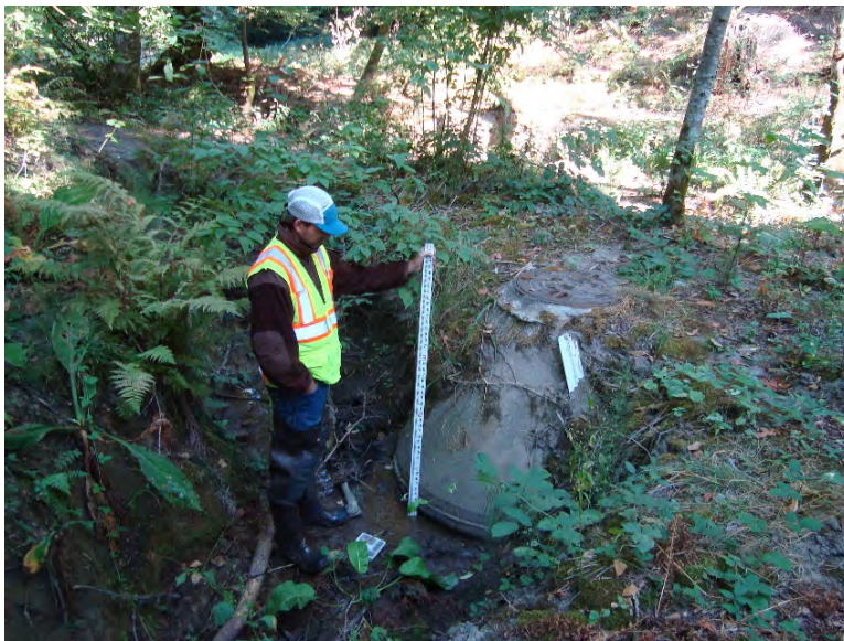
Photo 12. Side channel incision and erosion around sanitary sewer manhole.
