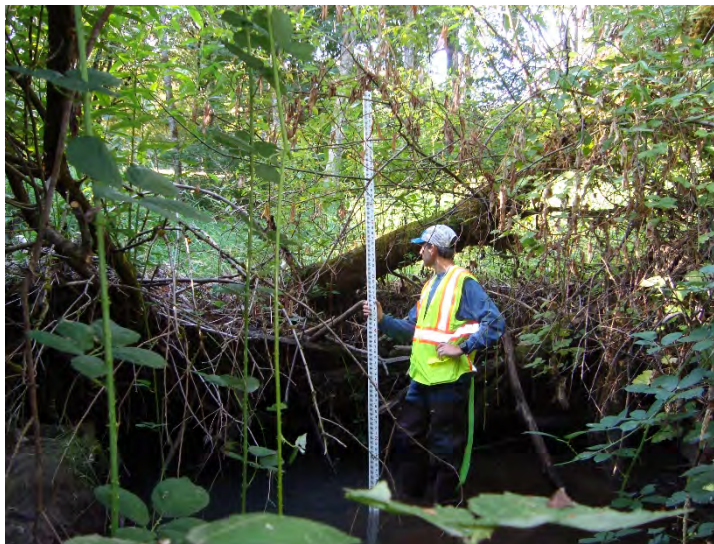
Site location: Between SW 55 th and SW 56 th , near I-205 Photo number: S2-4 Description: Channel spanning debris blockage, ~4' above channel bed, looking south and upstream
