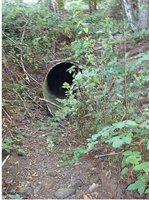
Site location: Culvert at SW Alsea Ct. Photo number: H3-29 Description: Looking downstream, upstream of SW Alsea Ct. Dry channel.
