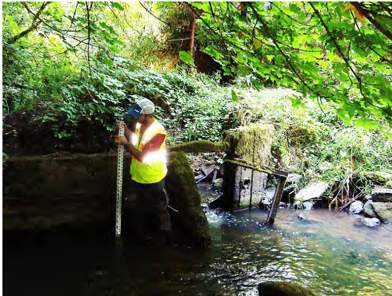
Site location: ~850' upstream of Tualatin, 20' upstream of culvert Photo number: S1-7 Description: Old 3' high concrete weir wall (2 ½' wide opening) with pool on downstream end. Weir is leaning downstream and sediment has deposited behind it on upstream side.
