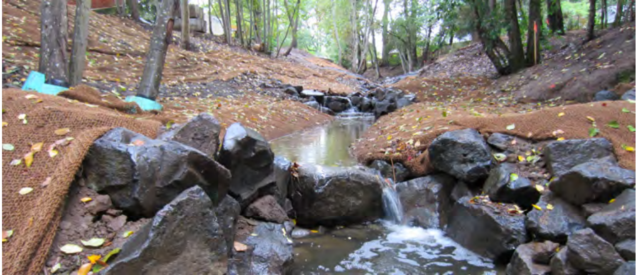
Photo 2. Otak photo of newly constructed Saum Creek channel in Chieftan/Dakota Greenway (c. 2013)
