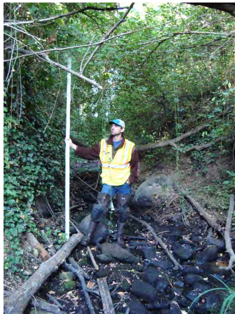
Site location: 30' upstream of Tualatin River Photo number: H1-2 Description: 1' - 2' rocks in channel, high water mark on bridge abutment corresponds to about 6' above channel bed in this location, steep gradient to mouth
