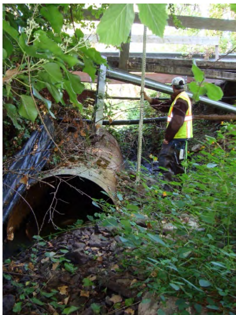
Photo 8. Culvert placed in debris from washed out bridge to convey Hedges Creek.
