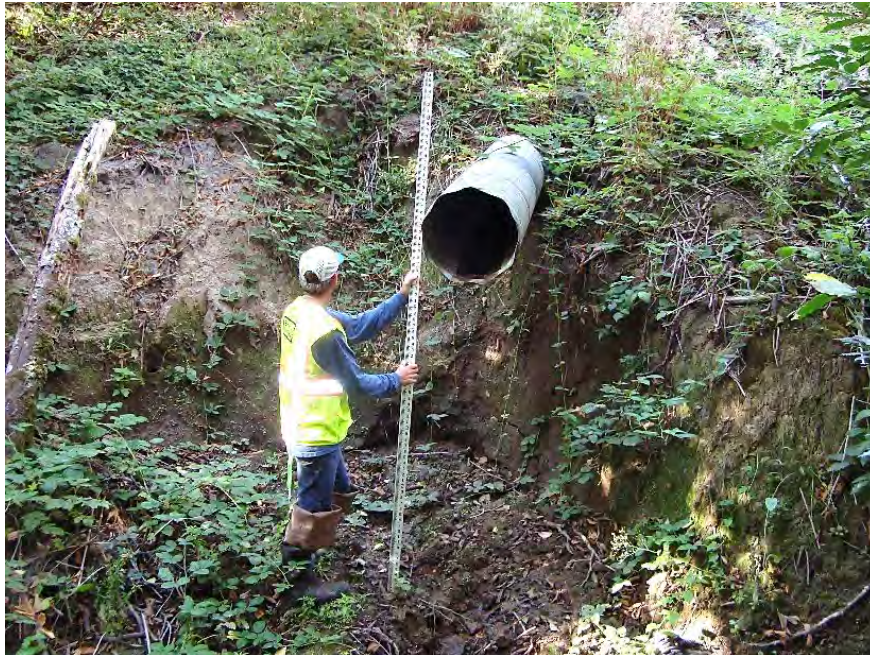
Site location: Downstream of SW Blake St. Photo number: S3-3 Description: Perched culvert- hillslope failure on left bank
