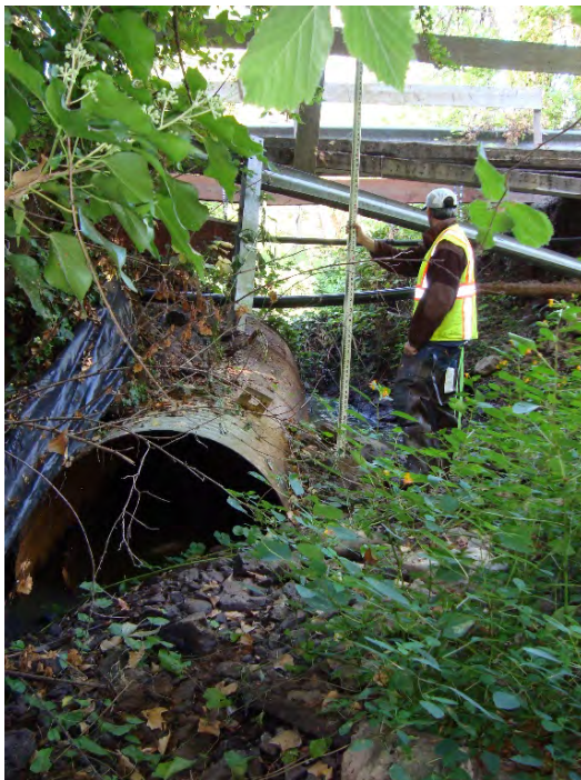
Site location: 500' upstream of Tualatin River Photo number: H1-12 Description: Looking upstream at culvert under washed out bridge amongst debris that has not been removed
