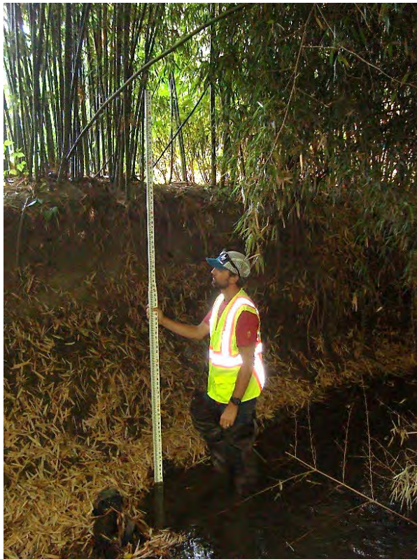
Site location: 30' upstream Photo number: S1-2 Description: 7' high vertical bank (right bank) unstable, bamboo
