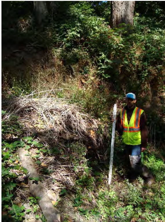
Site location: 1100' upstream of SW 105 th Ave. Photo number: H3-16 Description: Right bank slope failure, very wet
