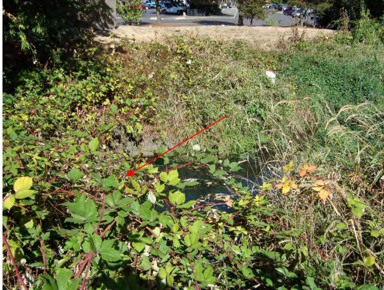
Site location: East side of SW SW Martinazzi Ave. Photo number: N3-1 Description: Looking downstream of SW Martinazzi Ave. where 48-inch diameter stormwater pipe enters Nyberg Creek (approximately where red arrow is pointing)
