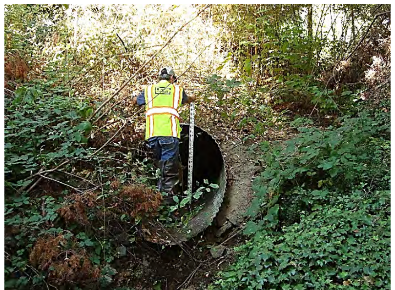
Photo 15. Perched culvert on downstream side of SW Alsea Ct.
