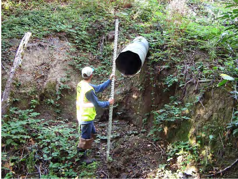
Photo 1. Hanging culvert on north side of Saum Creek Reach #3 in location of hillslope failure (September 2017)
