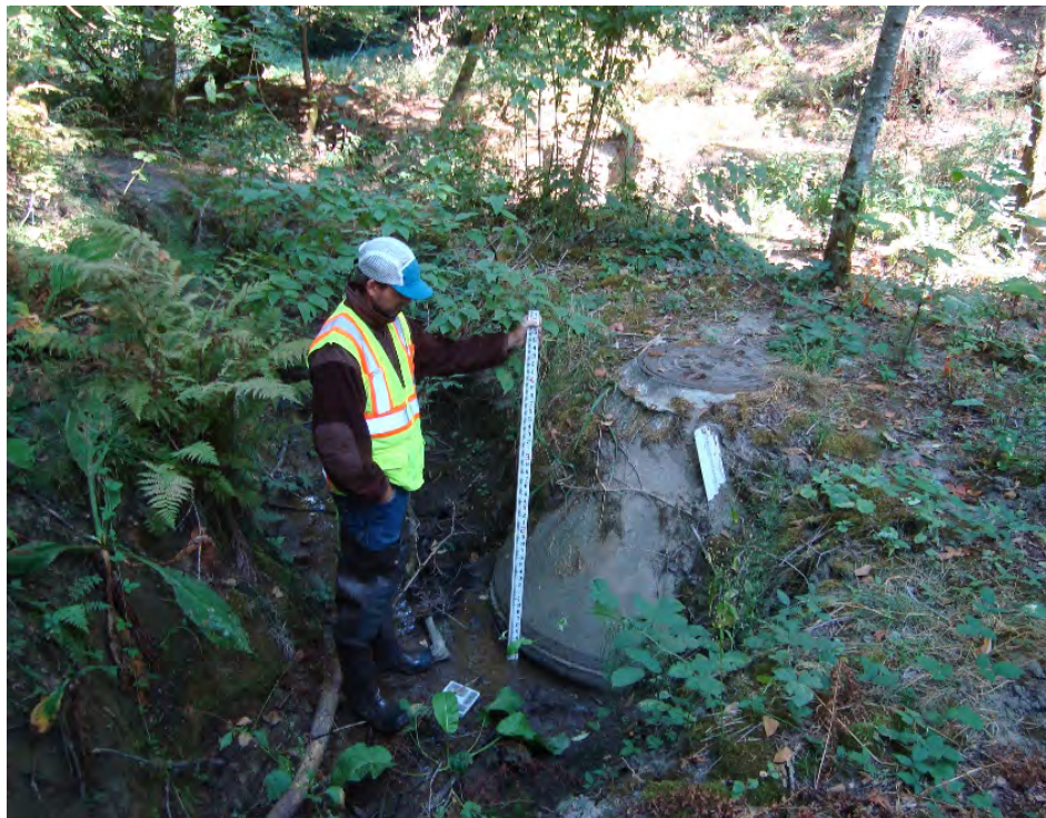
Image 1. Location ‘M’ exposed sanitary manhole and incised tributary
