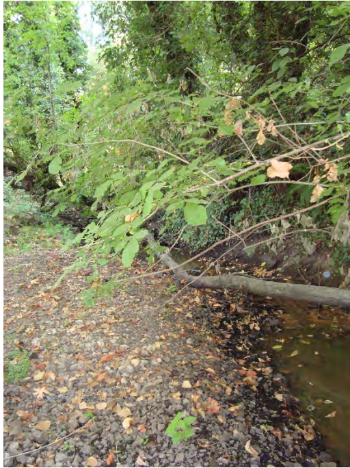
Site location: 500' upstream of Tualatin River Photo number: H1-11 Description: Looking downstream at debris and creek, right bank (outside bend) is downstream of culvert constriction (washed out) where flow is concentrated. This area is vulnerable to erosion.
