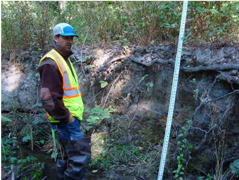
Site location: 900' upstream of SW 105 th Ave. Photo number: H3-14 Description: Outside bend erosion
