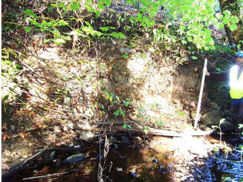
Site location: 175' upstream of SW 105 th Ave. Photo number: H3-5 Description: Left bank failure, missing wall segment adjacent to SW 105 th Ave., outside bend
