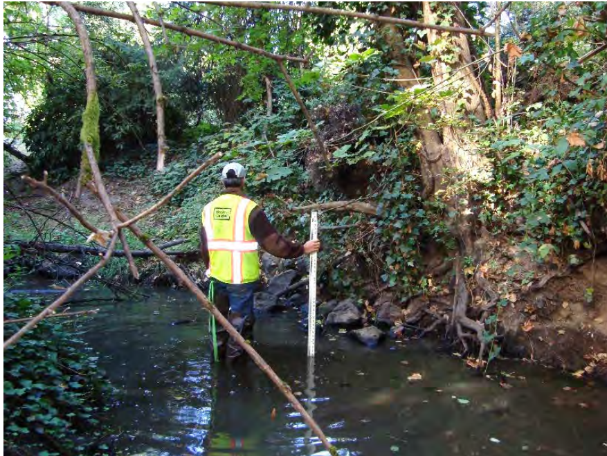
Site location: 450' upstream of Tualatin River Photo number: H1-9 Description: Looking upstream, bank armoring on left bank (right side of photo)
