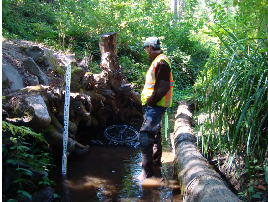
Site location: 950' upstream of SW 105 th Ave. Photo number: H3-15 Description: Restoration area, looking downstream. Left bank root wads, right bank anchored log
