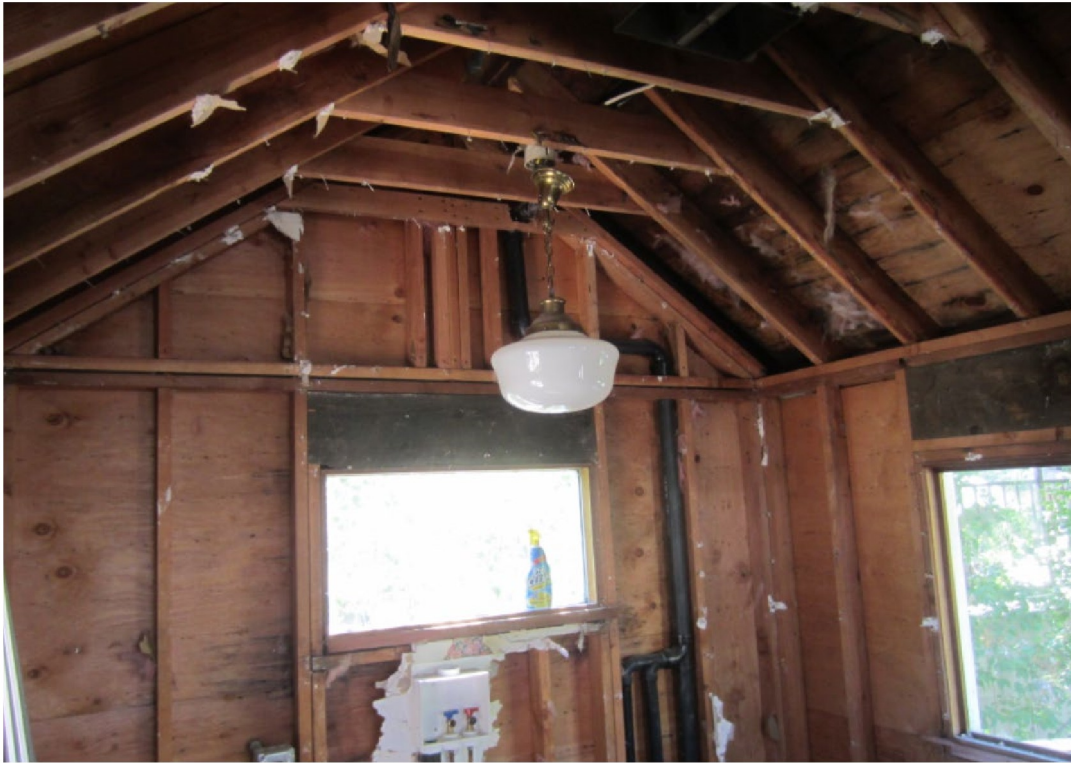
Figure 16 – Interior view of window (center) on second-story, western façade proposed for removal
