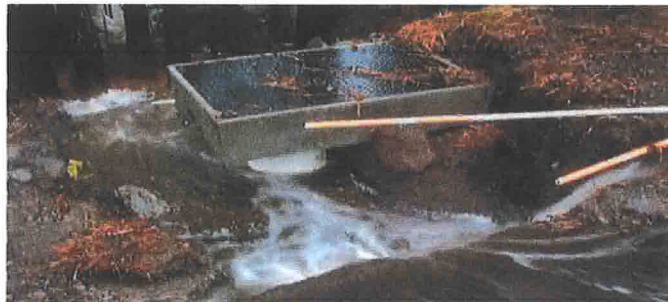
Utilities connecting West Donner to East Donner and located along Reed Avenue West compromised by runoff.
