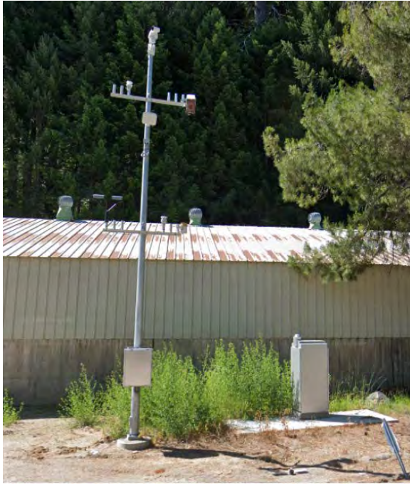
FIGURE 33. CALTRANS ITS STATION WITH TRAFFIC AND WEATHER SENSORS ON US 50 WEST OF ICE HOUSE ROAD
