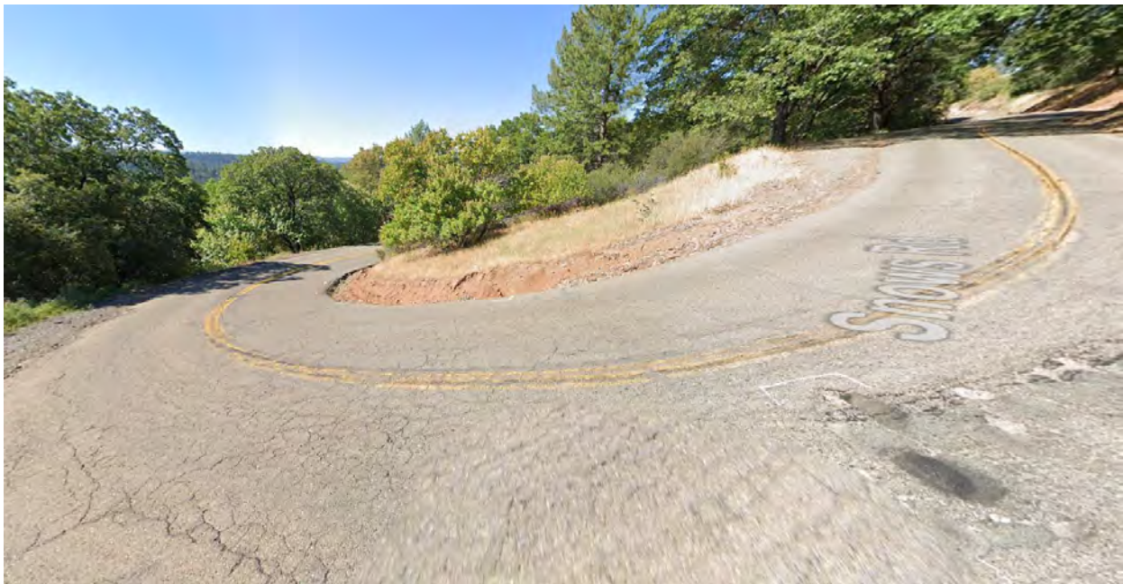
FIGURE 14: SNOWS ROAD WITH NARROW LANES, STEEP GRADE AND SWITCHBACK CURVE
