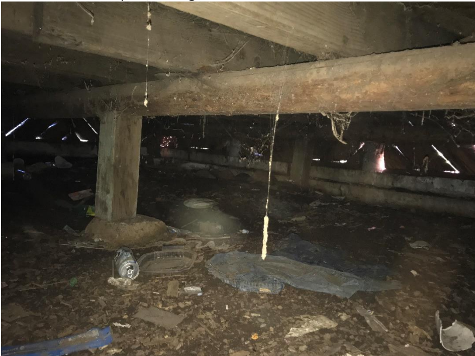
Picture 13 – shifted post/footing
