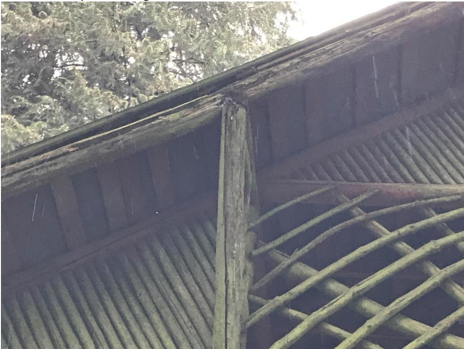
Picture 6 – dry rot damage
