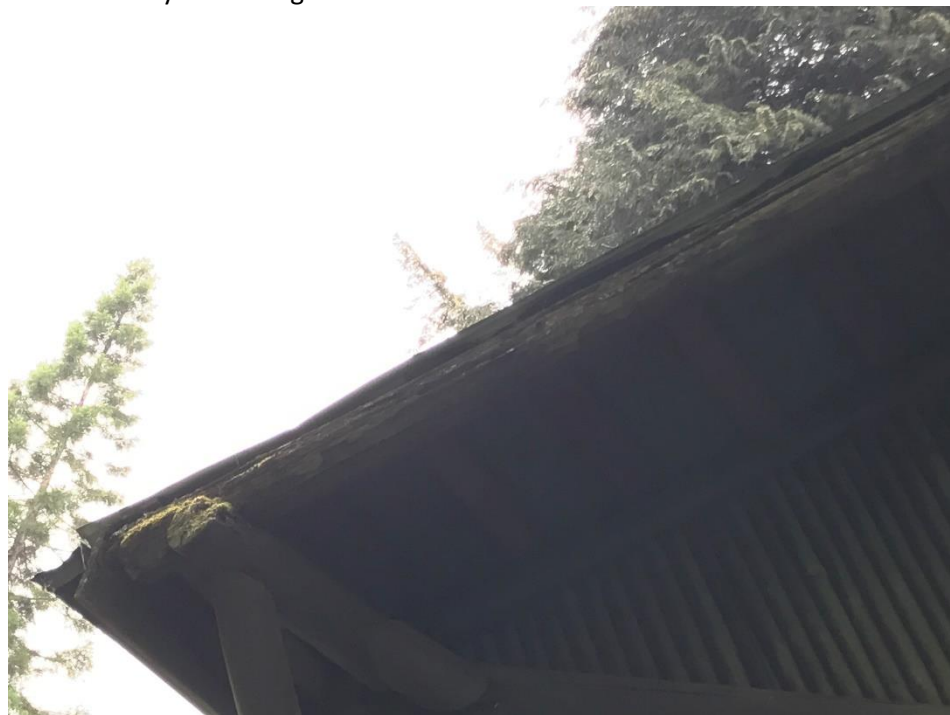
Picture 8 – dry rot damage
