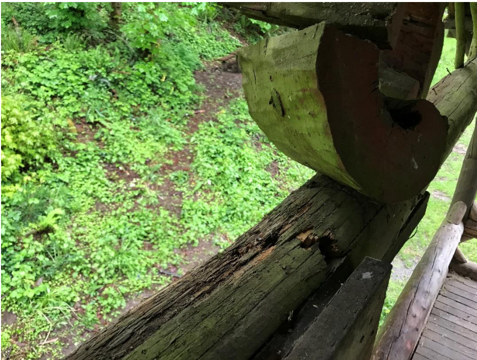
Picture 2 – Broken main member
