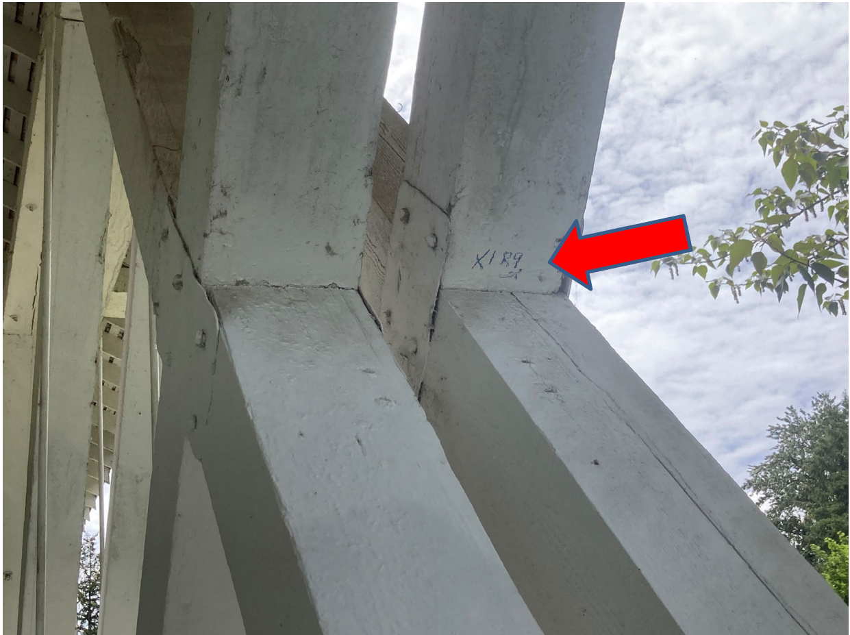
Figure 4– Downstream L3U4 (Left) 9" of Major Decay
