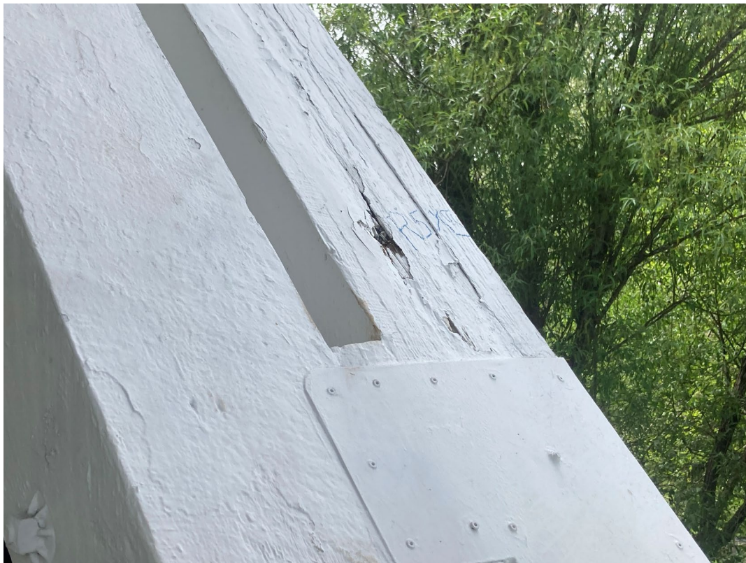
Figure 6 - Downstream U6L7 (Left) 5" Moderate Decay
