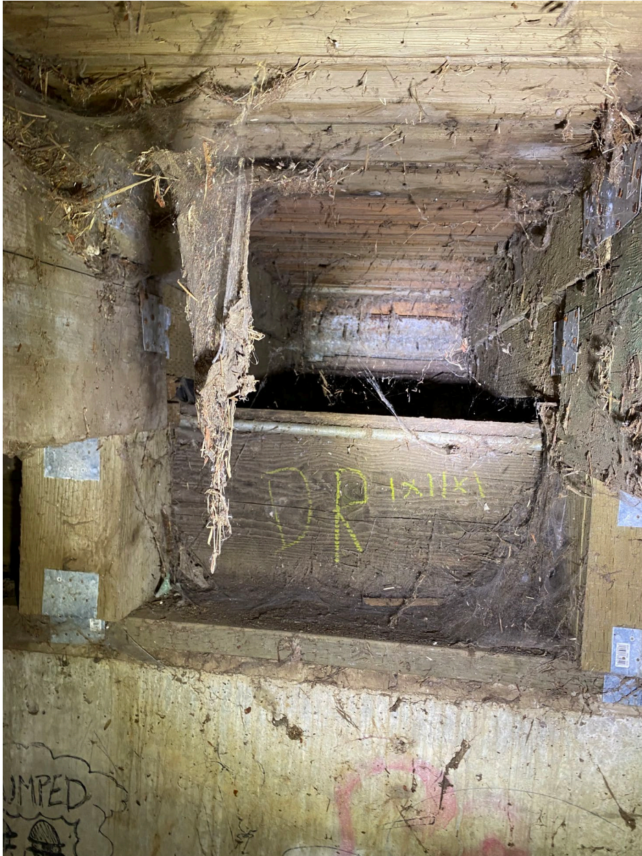
Figure 13 – Bent 1 backwall is a 1" shell with 11" of decay.
