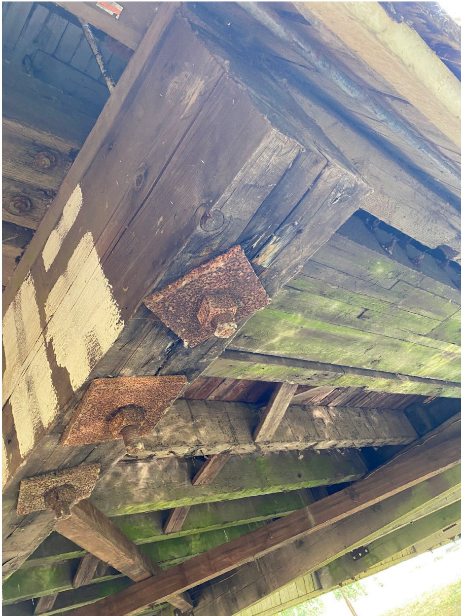
Figure 9 – Pitting on tie rod anchors
