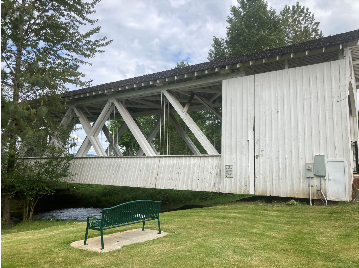
Figure 15 – Outside paint condition
