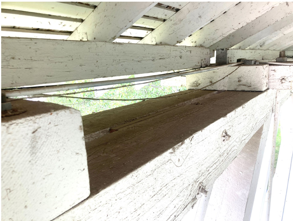
Figure 3 - Unpainted top chord
