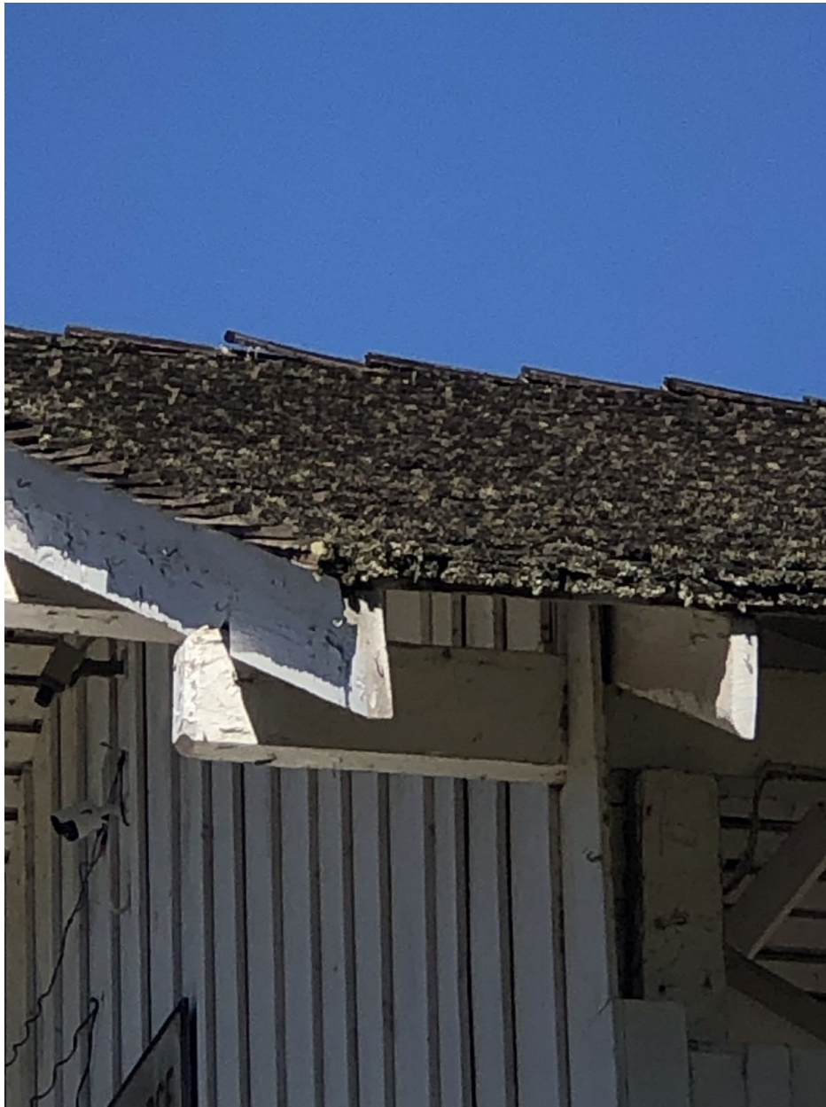
Figure 2 – Cedar shake roof should be replaced soon.
