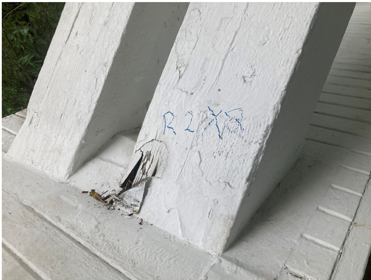
Figure 5 – Downstream L3U4 (right) 2" of minor decay
