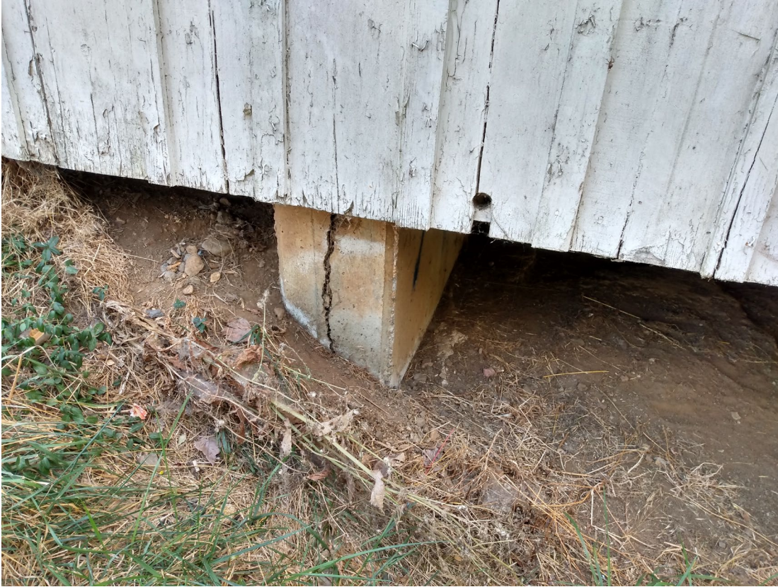
Figure 14 – Crack present in Bent 2 appears stable but should be monitored.
