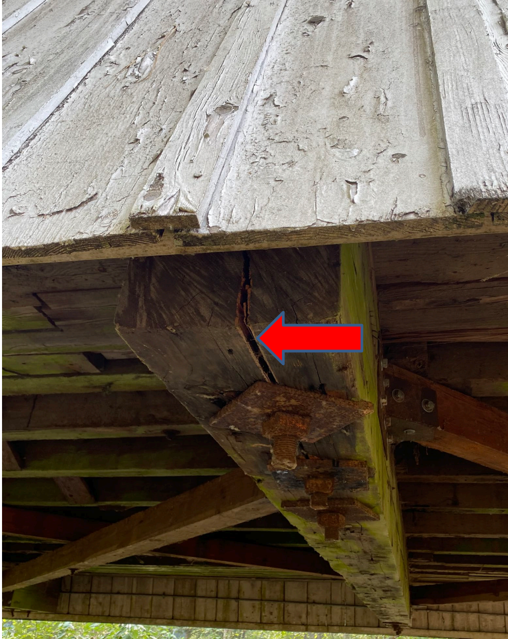
Figure 8 – Split at end of Floor Beam 3
