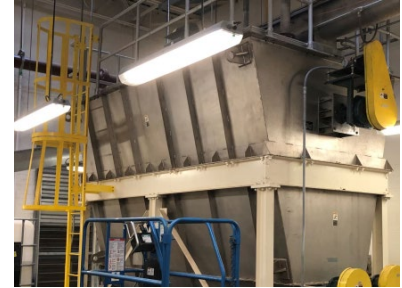
Sludge dryer at Lititz, Pa.
